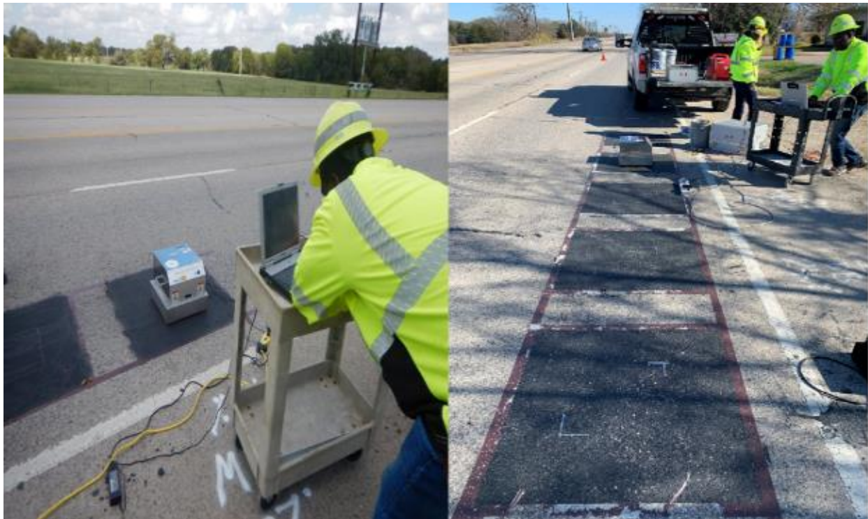
Figure 34. Before and After Traffic Passes of UTSS Surface Evaluation on SH 21.
