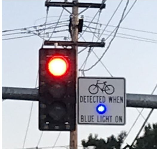
Figure 3.3: Blue detection confirmation light embedded in supplemental sign
