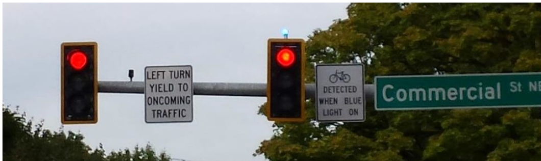
Salem, OR Commercial and Union Streets Blue Confirmation Light and Explanatory Sign (ODOT)
