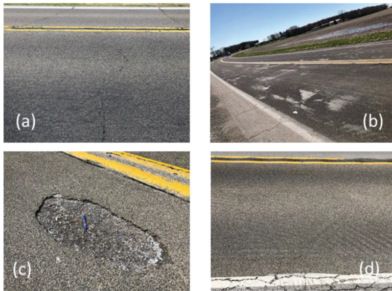
Figure 3.3 Most common early HFST distresses: (a) cracking, (b) aggregate loss, (c) delamination, and (d) surface wrinkling.
