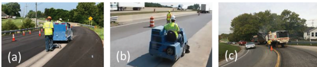
Figure 3.1 Photos of surface preparation operations: (a) shotblasting, (b) sweeping, and (c) scarification.
