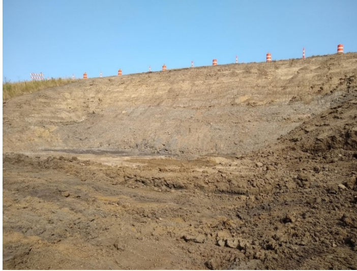
Figure 5.2 View of the slope with loose materials removed (Note: The total height is about 30 ft.)
