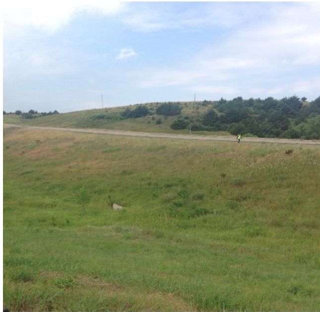
Figure 3.1 Verdigre slope at Highway 84 (Song et al., 2018)
