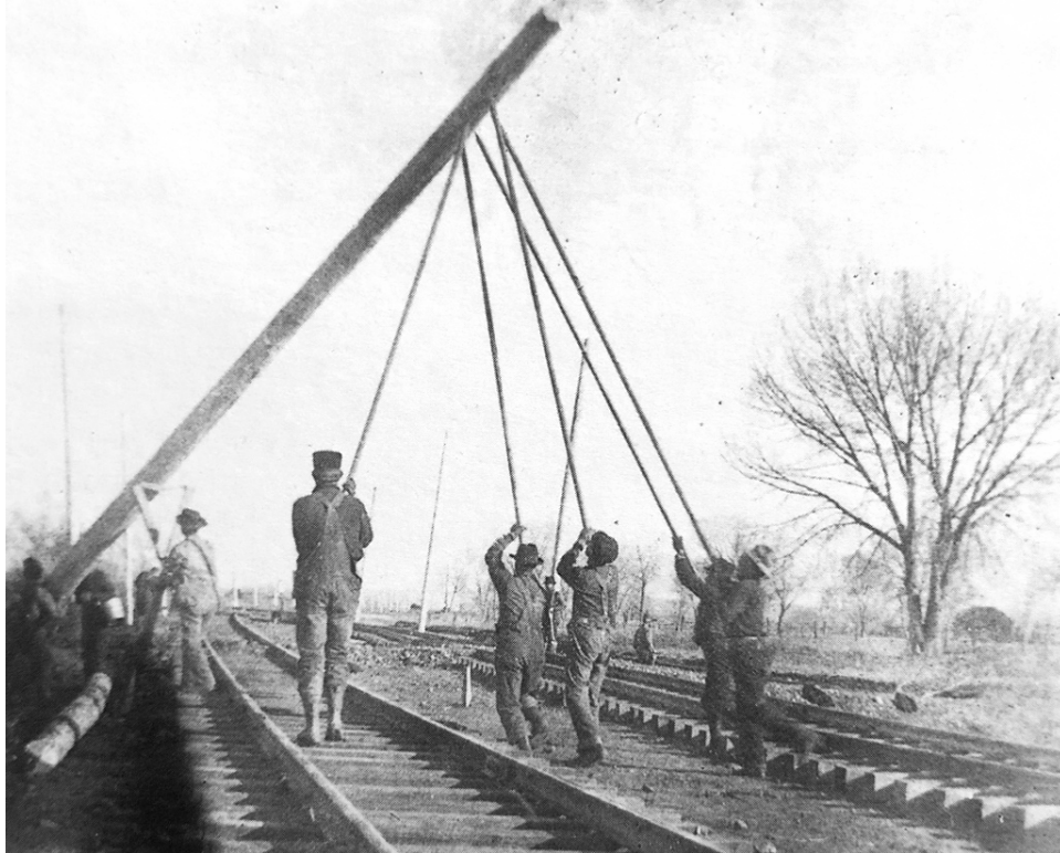
Figure 107. Crews erecting poles to support the catenary wire on the route to Golden. 515 It was common practice during the first part of the twentieth century for the poles to be painted white. 516
