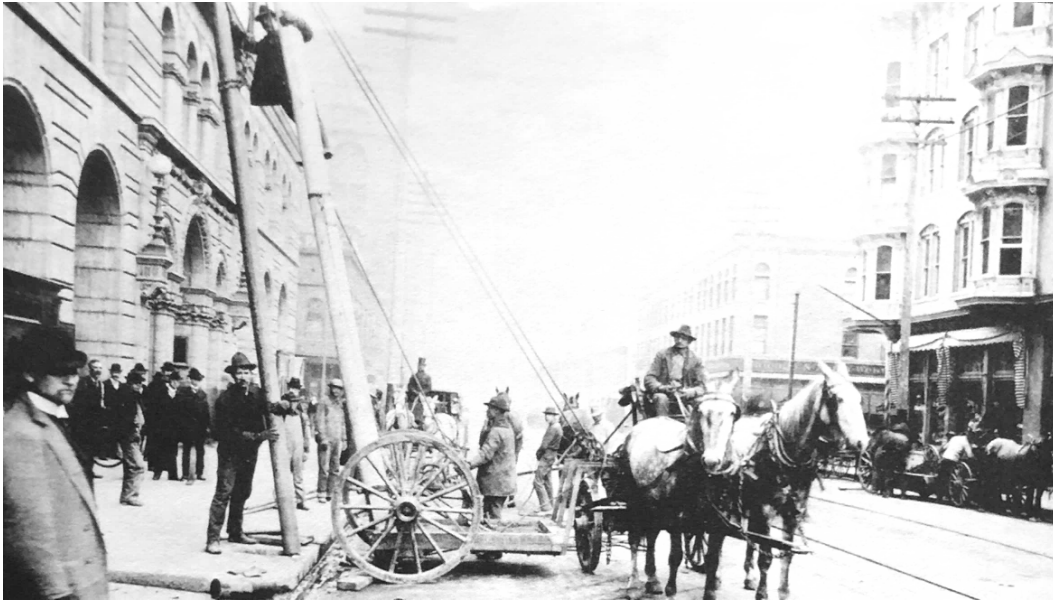
Figure 60. Erecting poles at the corner of 17th and Stout Streets for the conversion to electric traction. 310
