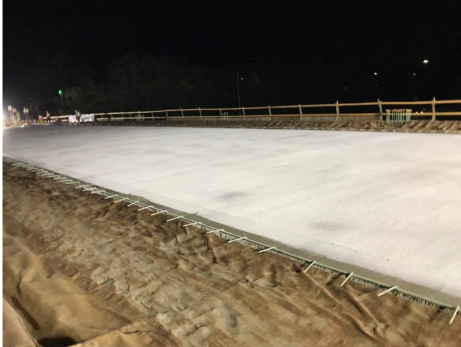
Figure 2.10: Finished IC-LC-HPC-4 Deck Showing Spots of Uneven Curing Compound Application
