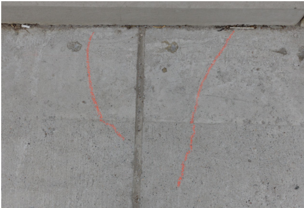
Figure 3.1: IC-LC-HPC-1 Typical Crack Pattern
