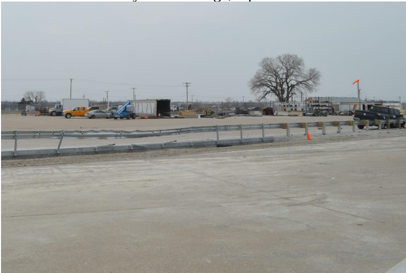
Overall System Damage, Upstream Behind View
