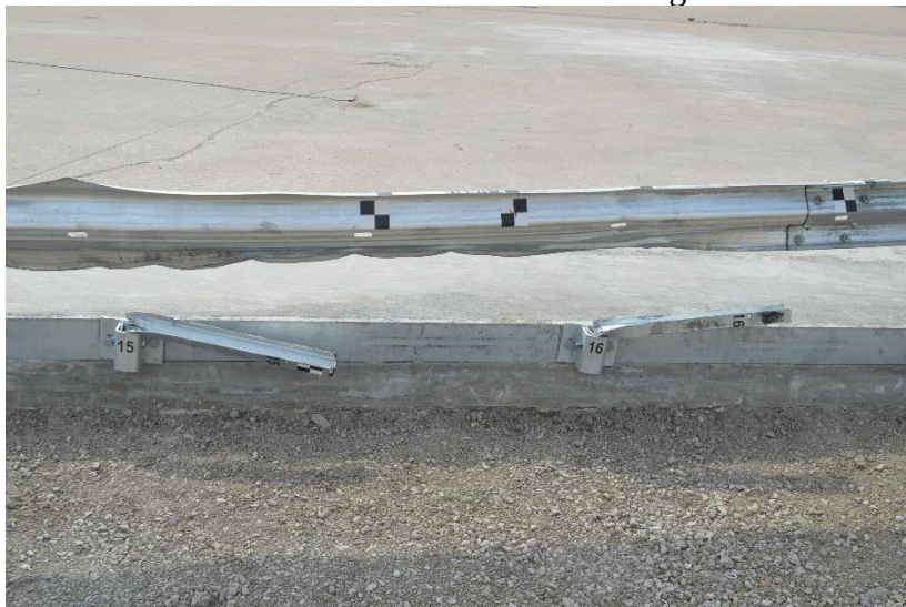
Post Nos. 15 and 16 Rear Damage
