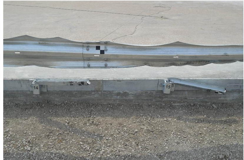
Post Nos. 14 and 15 Rear Damage
