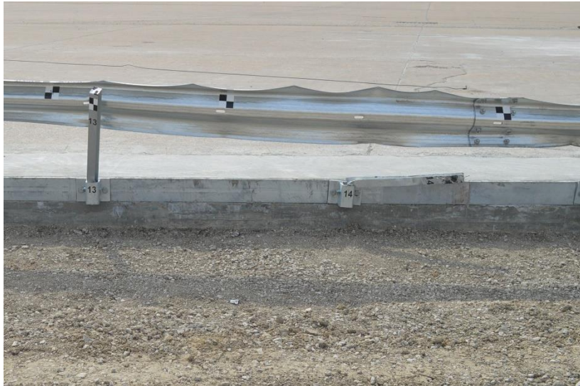
Post Nos. 13 and 14 Rear Damage
