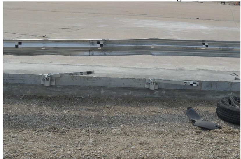
Post Nos. 16 and 17 Rear Damage
