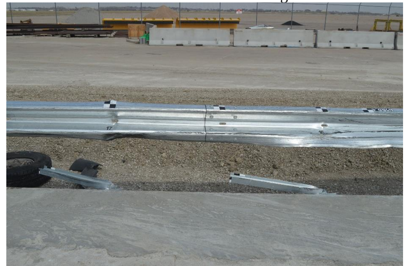
Post Nos 16 and 17 Damage
