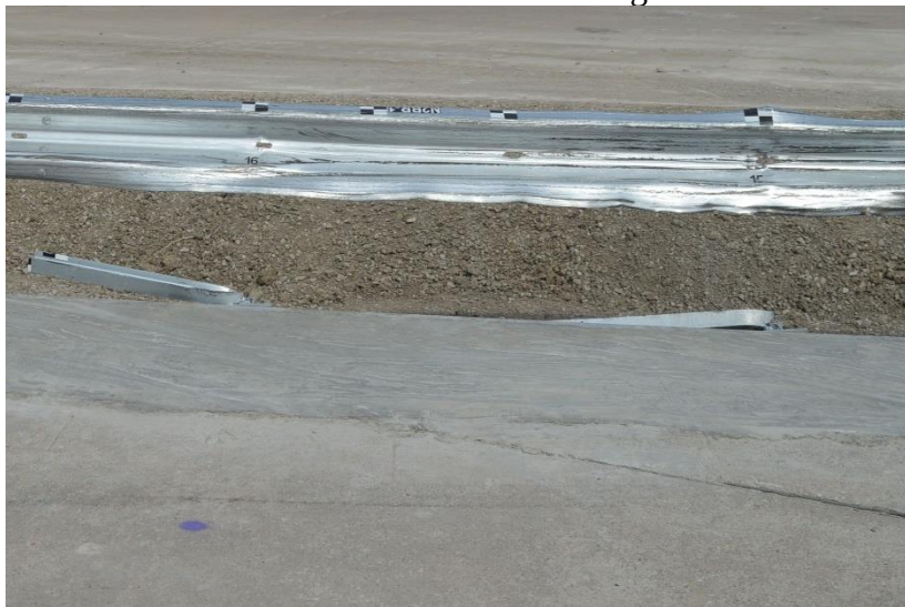
Post Nos. 15 and 16 Damage
