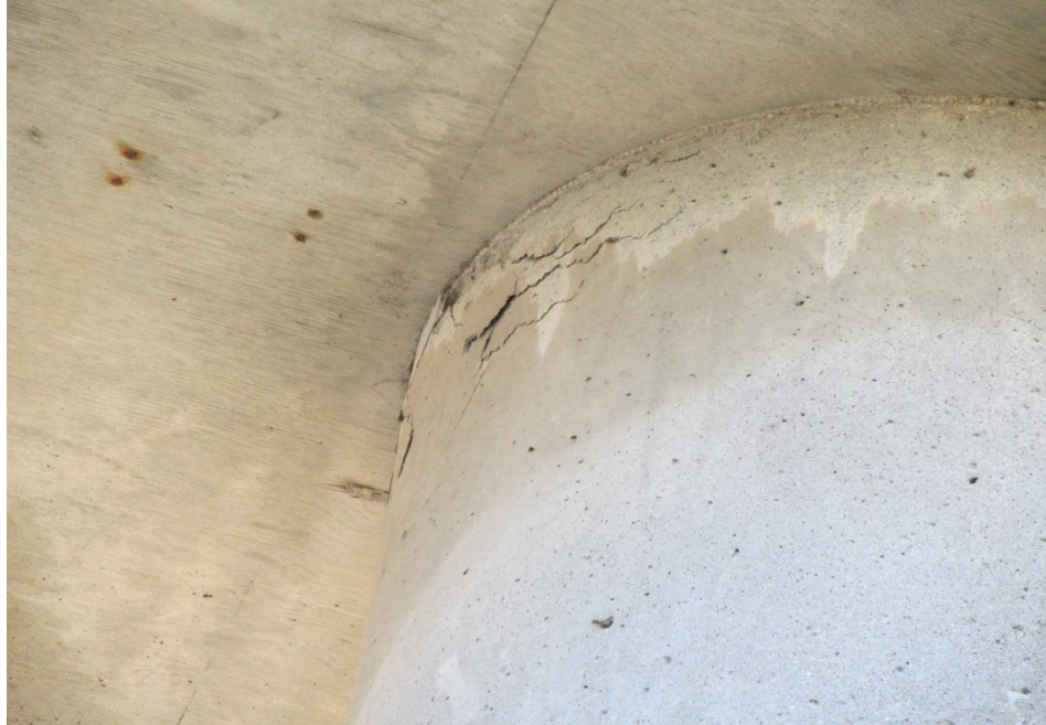
Figure 5.10: Concrete distress at top of the pier
