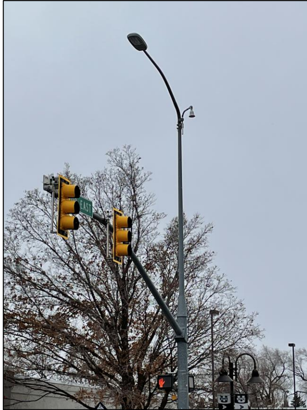
Figure 3-11 Overhead street light at a signalized intersection
