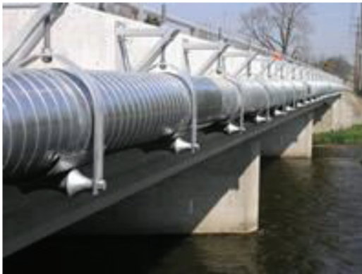
Figure 4.3 Conduit crossing a bridge (GF Urecon, n.d.).
