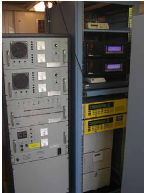
Figure 1. Hagerstown—The HA-NDGPS Broadcast Station Rack Figure
