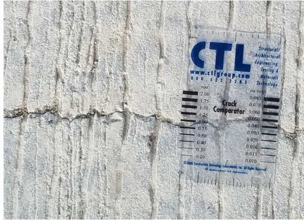
Figure 24. Crack width comparator for surface crack width measurement.
