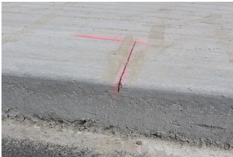
Figure 9. Saw-induced transverse cracks that are 2 feet long and 2 inch deep.
