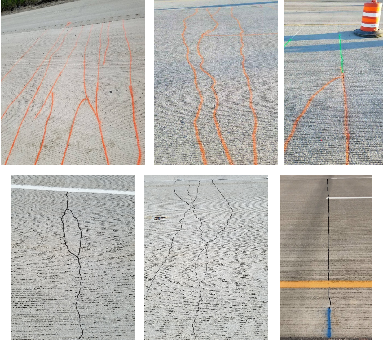
Figure 28. Complex Y-cracking with cluster cracks (top - left), cluster cracks showing three closely spaced transverse cracks (top-middle), Y-shaped crack (top-right), divided crack (bottom- left), complex y-crack (bottom-middle), straight transverse cracks seen in section 2 (bottom right).
