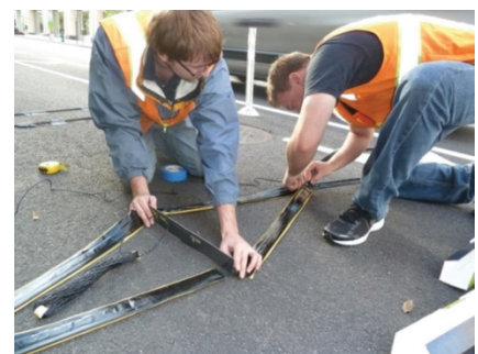
Figure 11: Technicians installing temporary inductive loop detectors (Source: Katie Mencarini, Toole Design Group)
