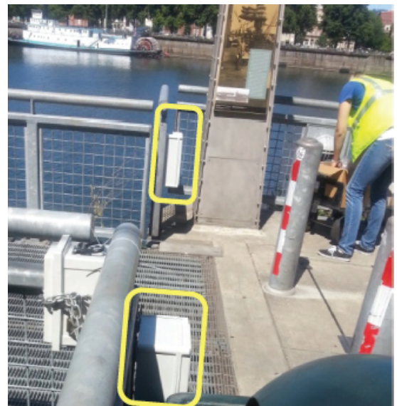
Figure 15: Completed radio beam counter installation. Source: Karla Kingsley, Kittelson & Associates, Inc. (Ryus et al., 2014b).
