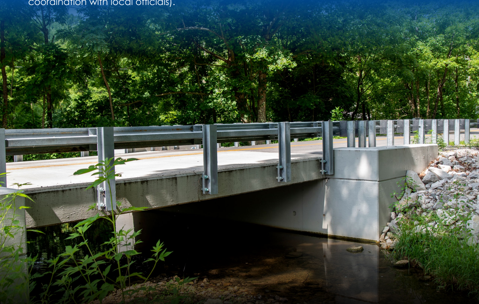
One of more than 260 bridges that have been replaced as part of the Bridging Kentucky program.
