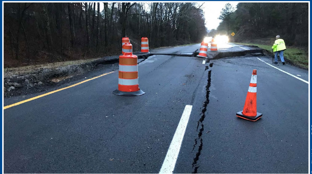
Initial slope movement closing US-231 due to massive landslide in Lacey's Springs, Alabama.
