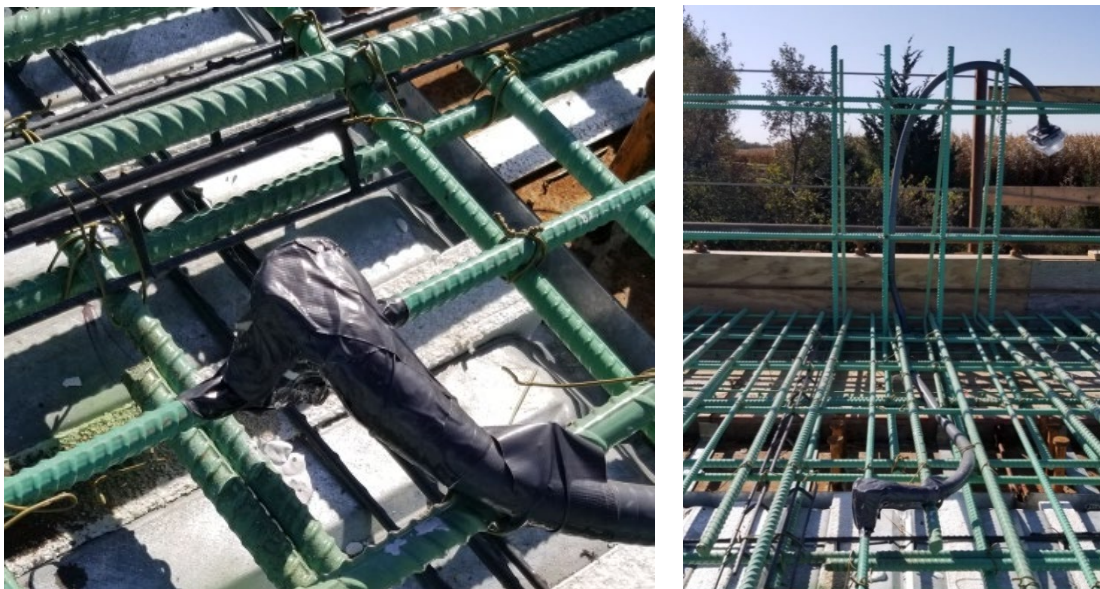
Figure 39. Valparaíso Bridge Instrumentation: (a) gypsum seat attachment of the ultrasonic transmitter wrapped in duct tape; (b) Sensor cable is protected inside a protective duct and ran to the side of the bridge
