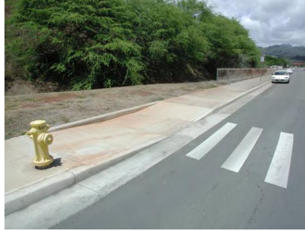
This is a bad example of a missing detectable warning.
