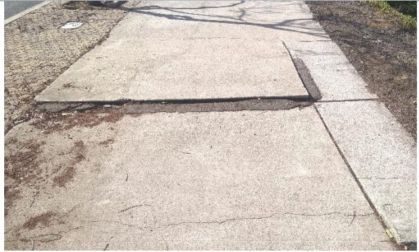
This picture shows a sidewalk with a change in level, which is a pedestrian hazard.
