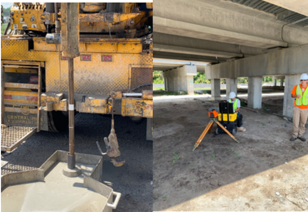
Figure 6-12 Images of SPT and PDM Setup for Wekiva Parkway Day 1 (Photos by Dr. Cosentino)
