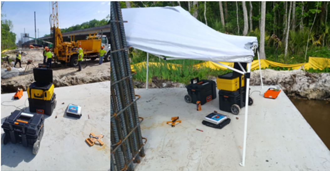
Figure 6-10 Images of SPT and PDM Setup for Dunns Creek (Photos by Robert Rogulski)
