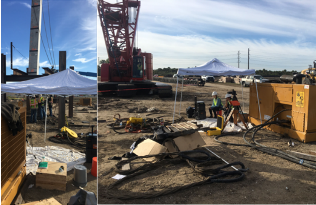
Figure 6-9 Images of Pile and PDM Setup for Ellis Overpass (Photo by Dr. Cosentino)
