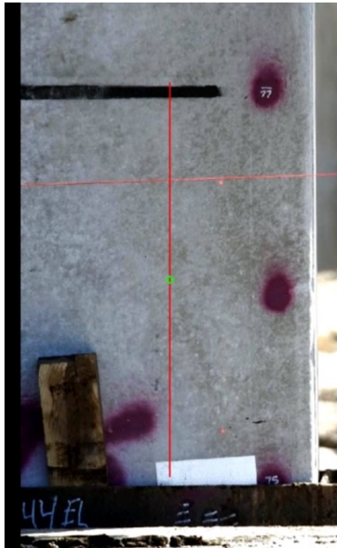
Figure 6-27 CMS Video Image from Dunns Creek Test Pile 10 at Pier 4 at 75- to 77-foot Pile Markings
