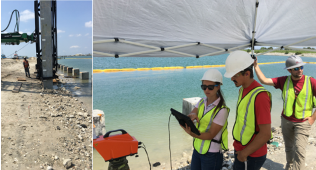
Figure 6-2 Images of Pile and PDM Setup for Port Canaveral Day 1 (Photos by Dr. Cosentino)
