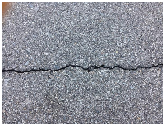
Figure 7- 1 Original image of a crack
