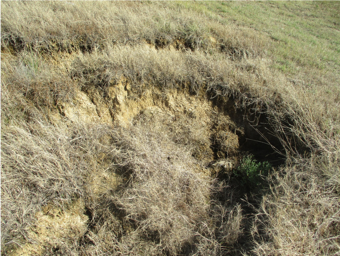
Figure 4.42 Soil Erosion at the slope surface at Slope 4
