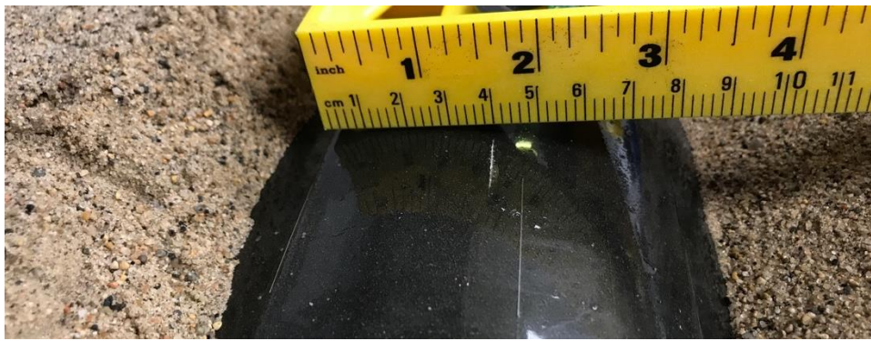
Figure 89. Distance measurement between crack and Sensor 1/Sensor 3.
