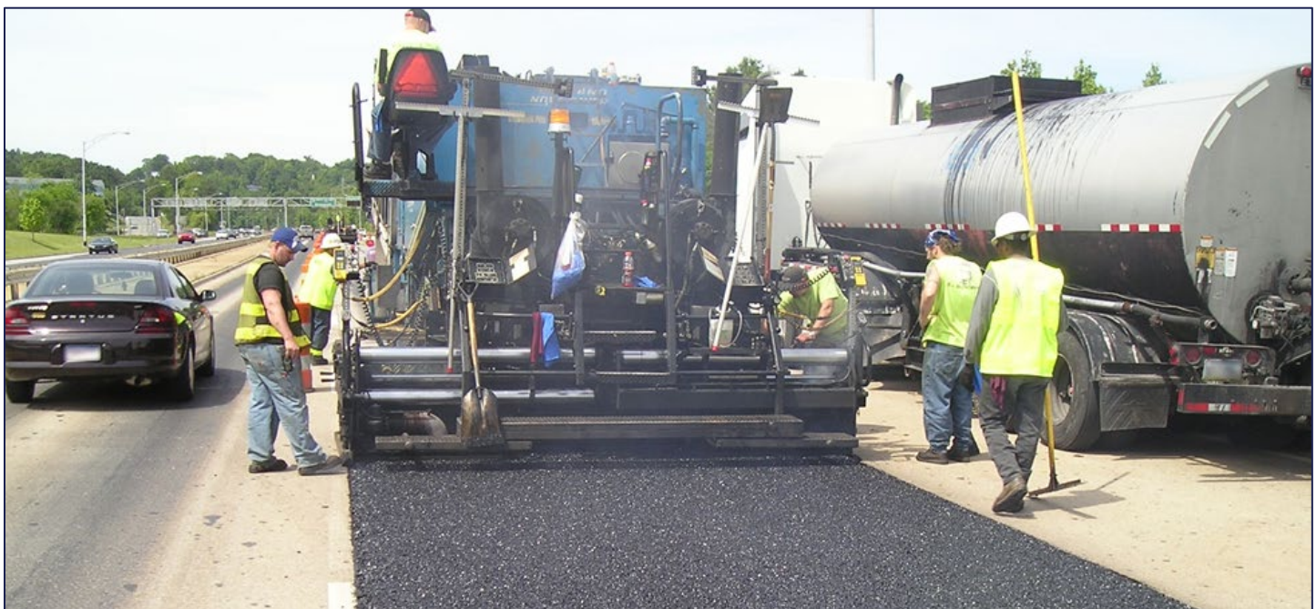
Crews place ultra-thin bonded wearing course. Source: National Center for Asphalt Technology
