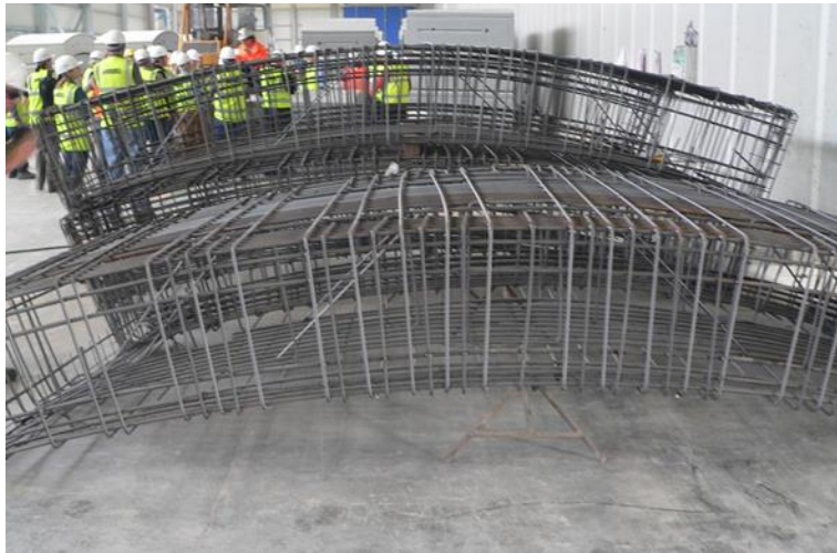
Figure 5-1: Steel rebar reinforcement for the Galleria Sparvo tunnel in Italy. Photo: FHWA.
