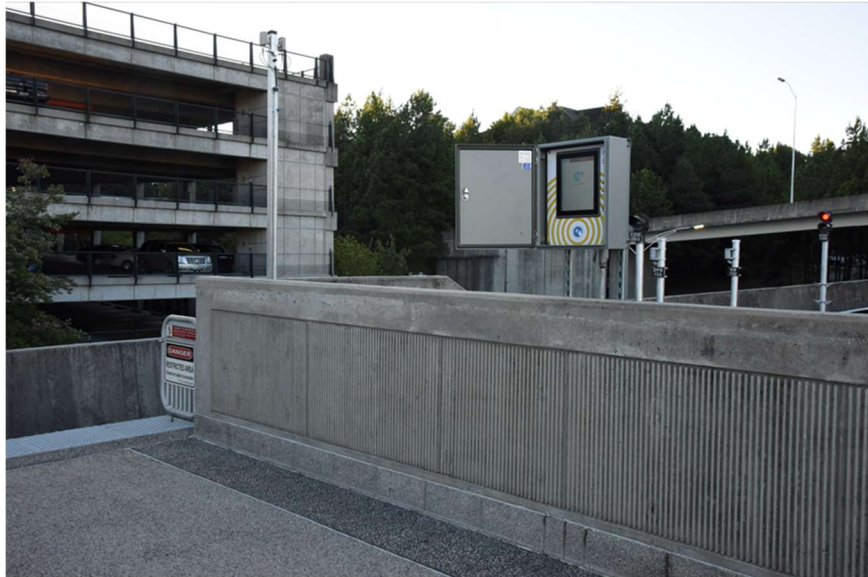
Figure 4 - Wayside Access Unit (WAU) at North Springs Station platform
