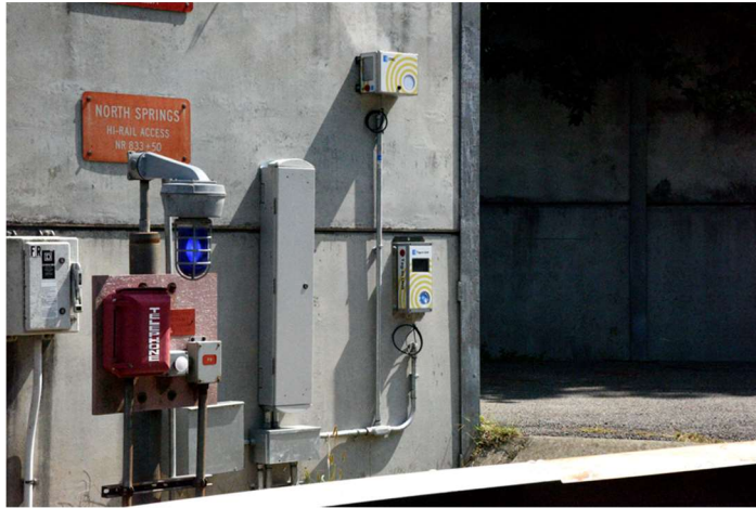
Figure 5 - Tag-In Unit (TIU) at North Springs Hi-Rail Access point
