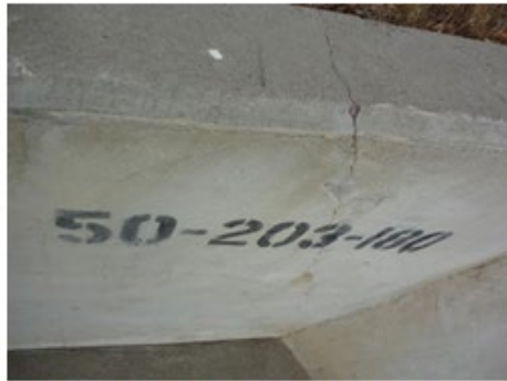
Crack through the Wall Thickness
