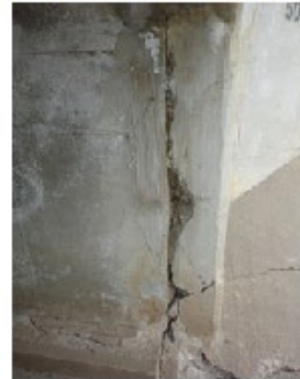
Cracking between the Culvert Wall and the Wing Wall Extension
