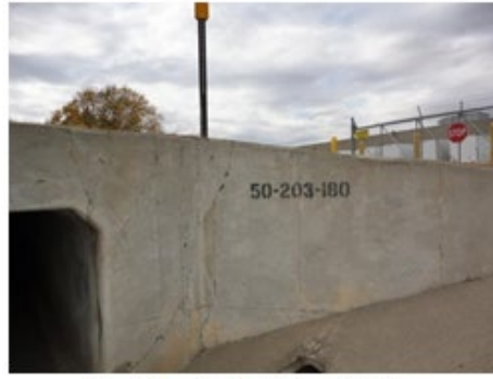
Cracking in the Wing Walls
