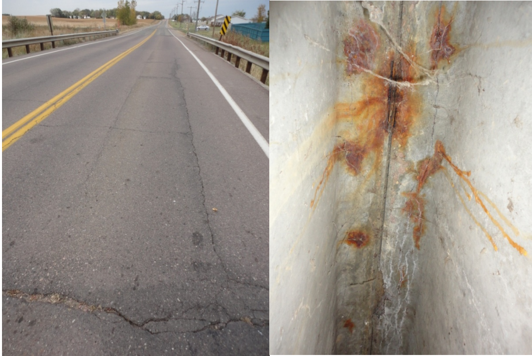
Figure3.5 Leaking joints and spalling of concrete
