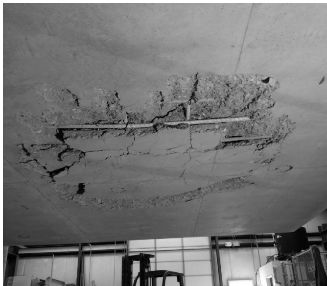
Figure 8.4.10 Bottom of HRC post-fatigue punching shear deck
