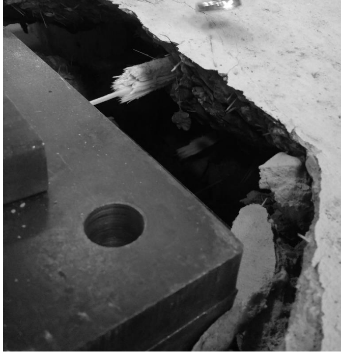
Figure 8.2.8 Shear rupture of GFRP bar
