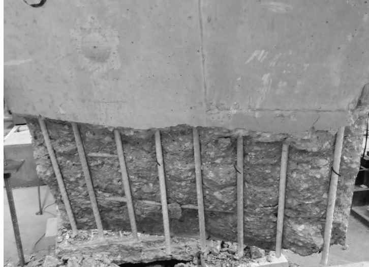
Figure 7.4.14 Bottom view of GFRP specimen after failure
