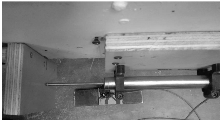
Figure 3.3.17 LVDT spanning crack at bottom level of deck
