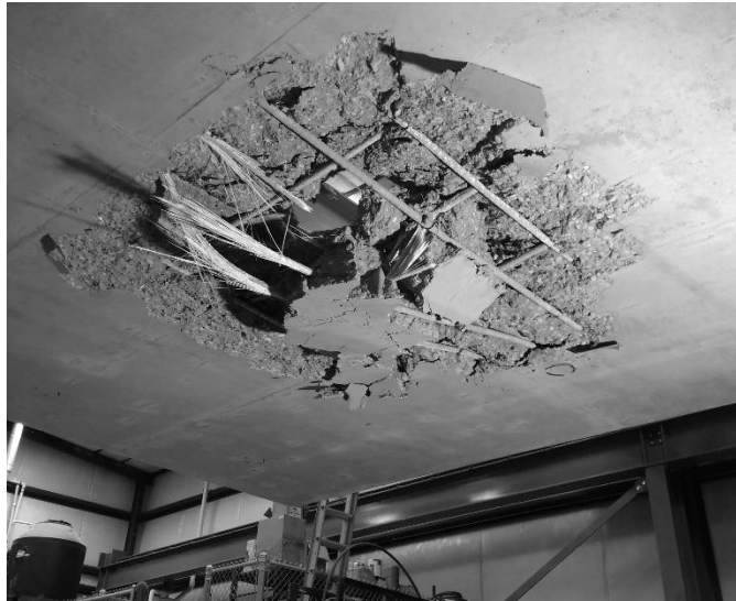
Figure 8.2.11 Bottom surface of HRC punching shear deck
