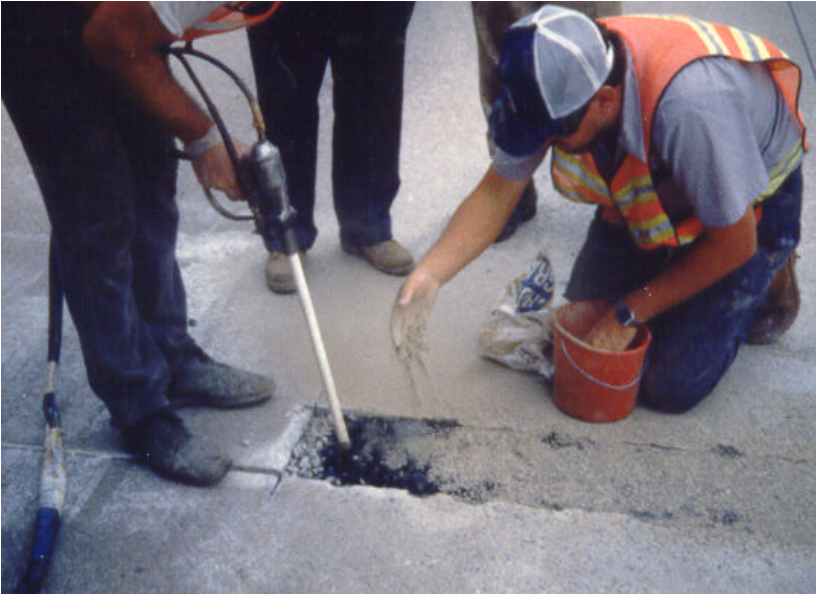
Figure 23. Pumping polymer into a patch that was prefilled with aggregate (cover aggregate also being placed).
