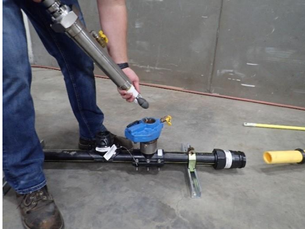
Figure 30 Stuffing Box with Mapping Tool Pipeline Entry
