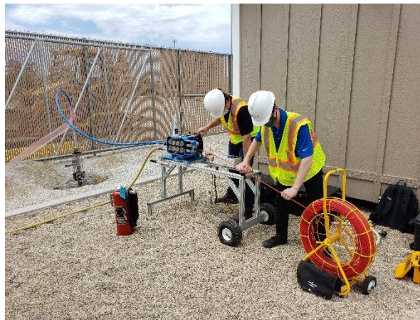
Figure 58 Operation of Live Natural Gas Pipeline Mapping System
