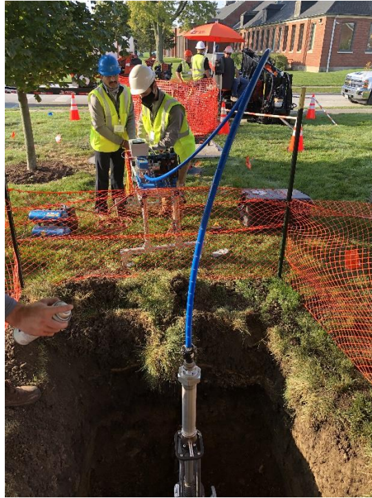
Figure 64 Photo of 3D Mapping Probe Demonstration in 4" PE Pipe.
