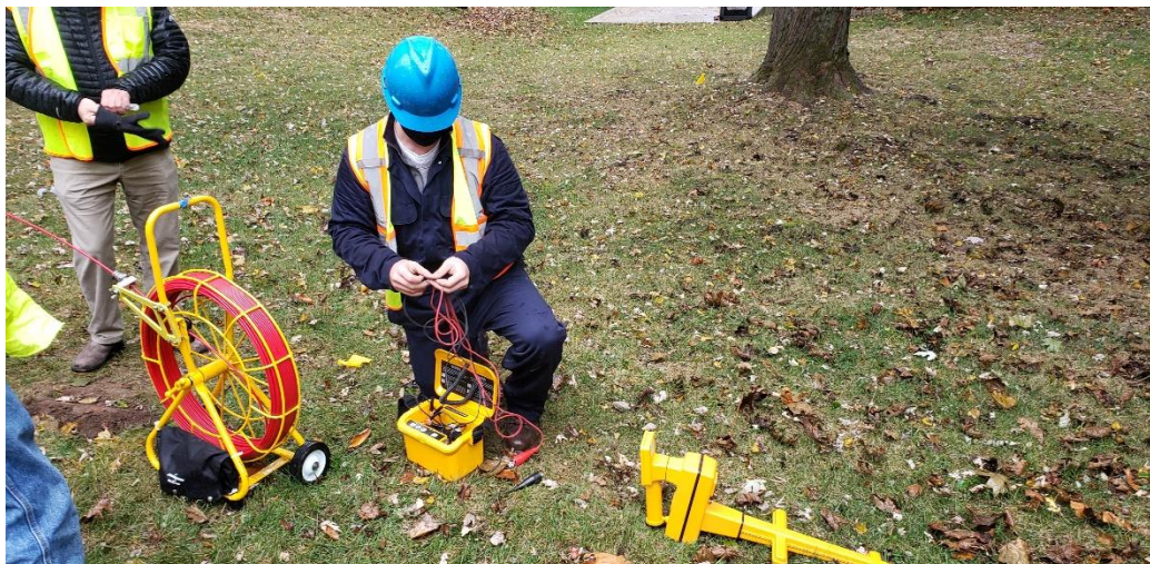
Figure 68 GNSS Geospatial Data Collection Via an Underground Energized Tracer Wire with a Surface Locator
