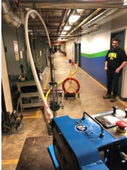
Figure 44 Evaluation of Mapping System and Operation of the Pneumatic Duct Rod Pusher
