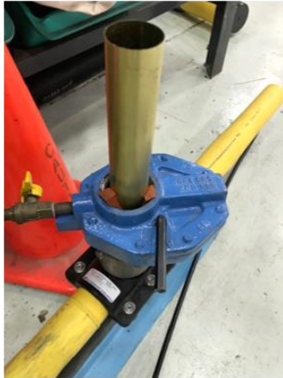
Figure 28 Pipe Access fitting
