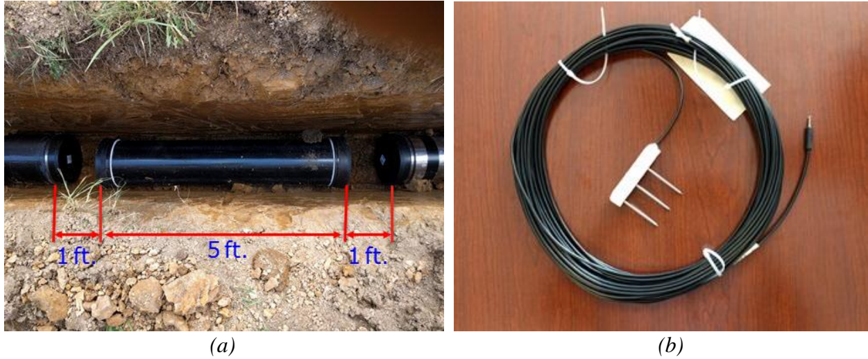
Figure 5-5: (a) Arrangement of pipes in the trench, (b) soil moisture and resistivity sensor
