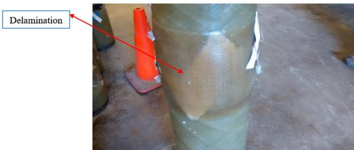
Figure 3-3: Delamination of wrapped butt joint
