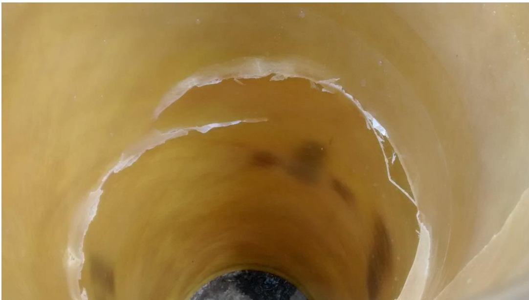
Figure 2-15: Damage to corrosion barrier
