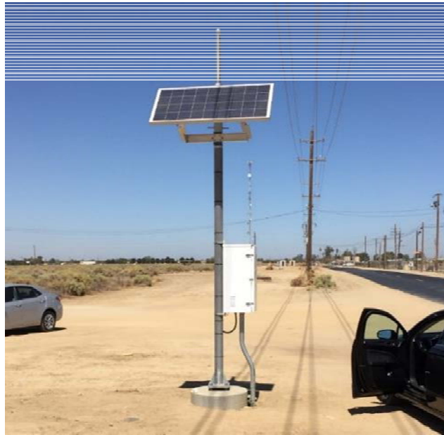
Figure 45: Solar Powered Enclosure in Place
