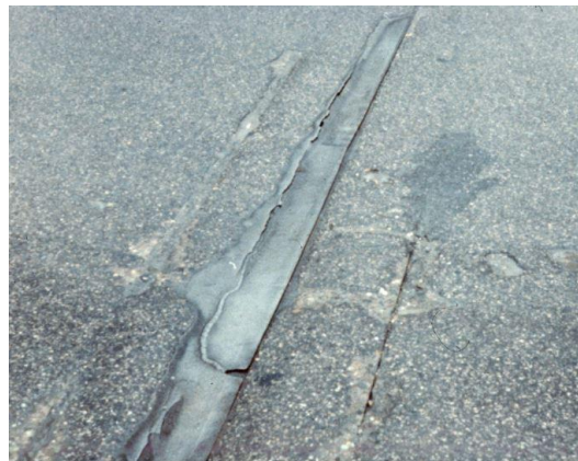
Figure 2.2. Sliding plate fused and separated from abutment
