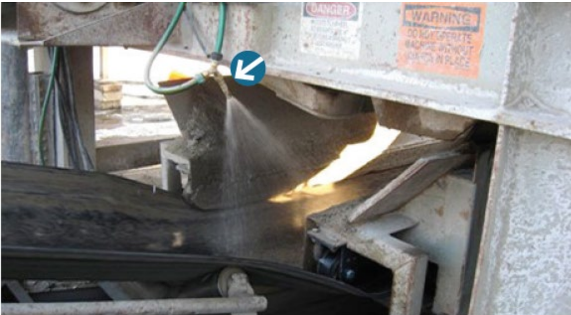
Figure 7.2 Spray Nozzle for Dust Control on the Aggregate Conveyor (Snyder, 2018)
