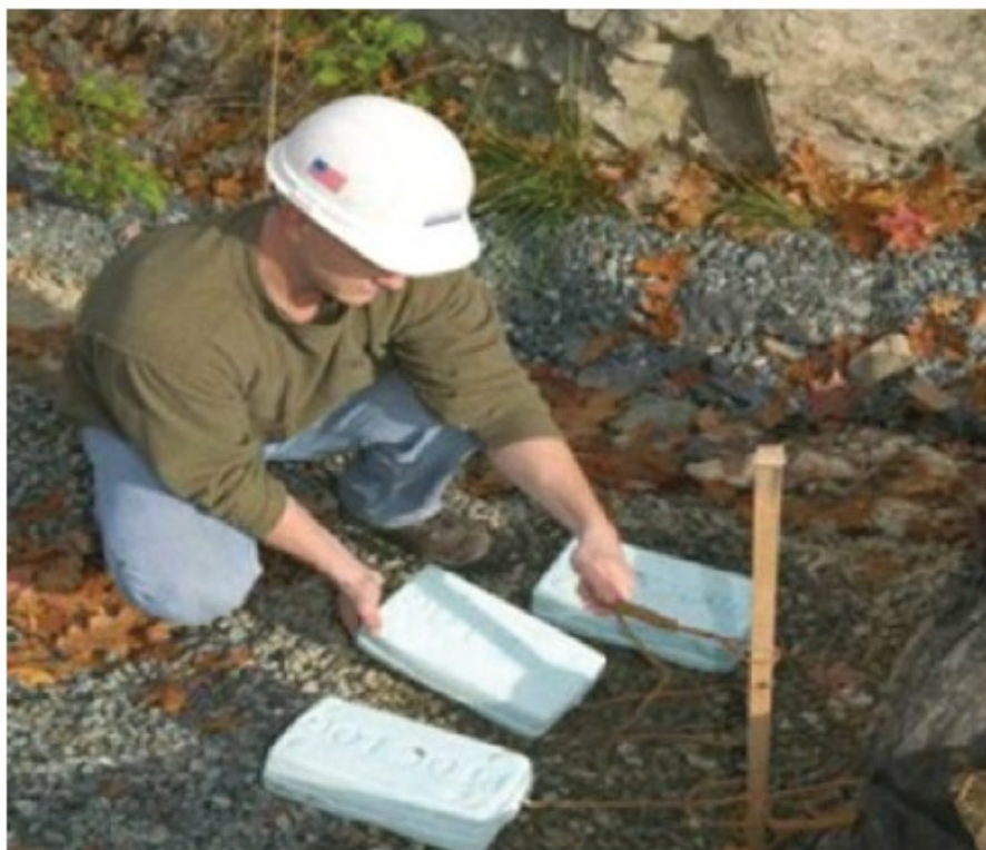
Figure 2.3: Floc Log Tied to a Wooden Stake in the Outflow Path (Cavalline, 2018b)
