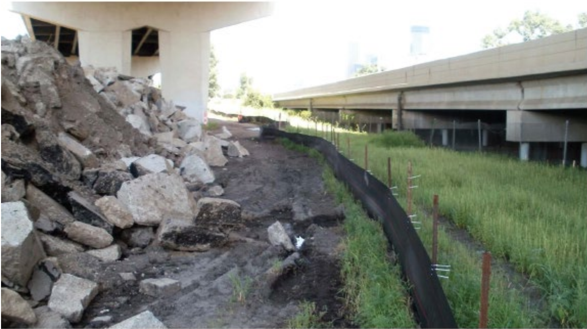
Figure 7.1 Demolished Material Stockpiled Beneath Bridge Prior to Crushing with Silt Fence and Vegetative Buffer Used (Snyder, 2018)
