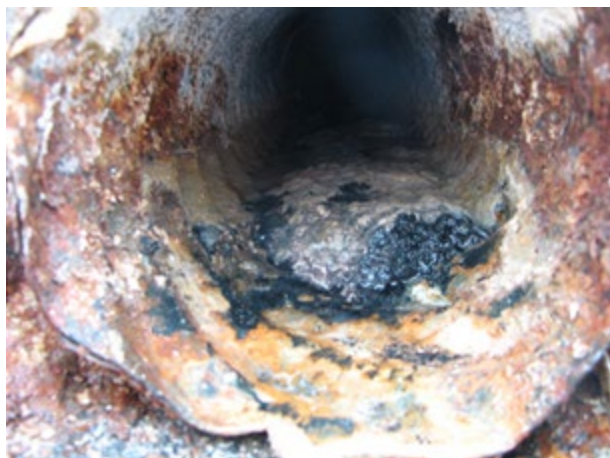
Figure 4.3: Underdrain Outlet Condition after 2 Years of Service, I-69 East of Flint, BFSA Base (MDOT, 2009)
