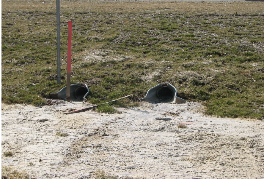
Figure 4.4: Underdrain Outlet Condition after 1 Year of Service, I-75 near Bridgeport, RCCA Base (MDOT, 2009)
