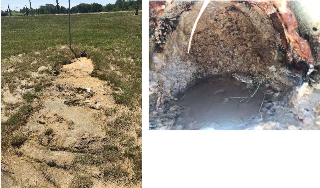
Figure 5.6 Underdrain Outlet at UniR-I75N-1 (RCCA Base, Year of Construction 2015, Age 5 Years)
