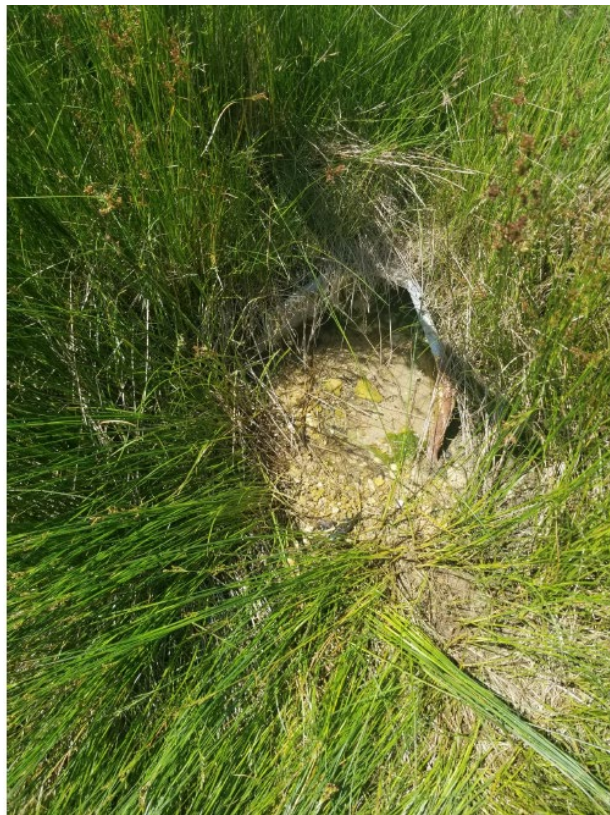
Figure 5.5 Underdrain Outlet at I96E-PH-1 (RCCA Base, Year of Construction 2011, Age 9 Years)
