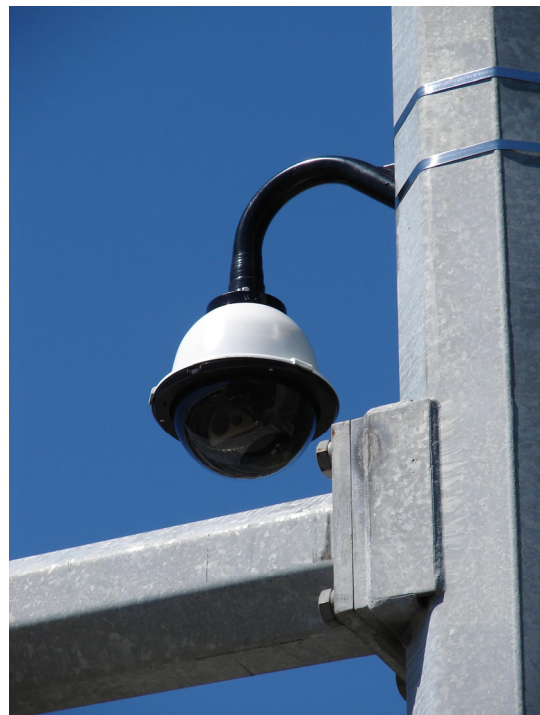
Figure 10. PTZ Camera on Signal Pole
