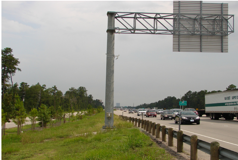
Figure 11. PTZ Camera and Sensor on a Sign Bridge
