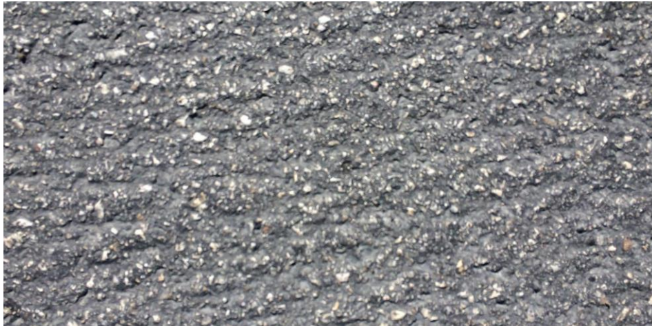
Figure 36. Photo taken from SH 151 test site 12 months after the milling
