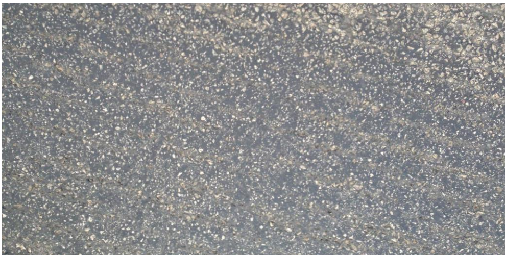
Figure 42. Photo taken from US 277 test site 12 months after the milling
