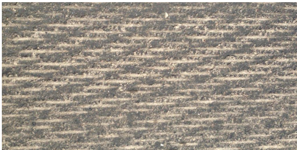
Figure 40. Photo taken from US 277 test site 3 months after the milling
