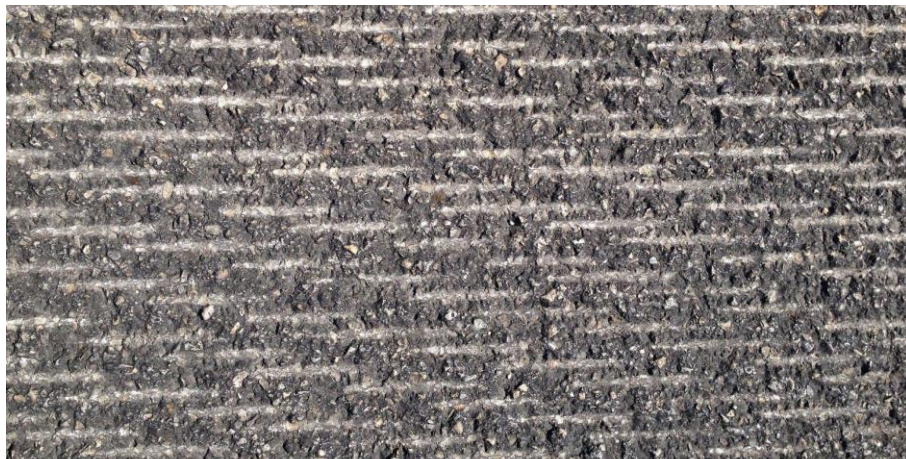
Figure 29. Photos taken from Wurzbach Parkway test site 6 months after the milling
