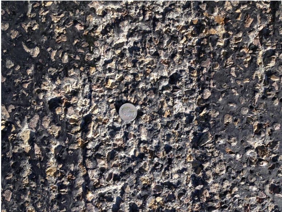
Figure 23. Photo taken from US 87 test site 6 months after the milling
