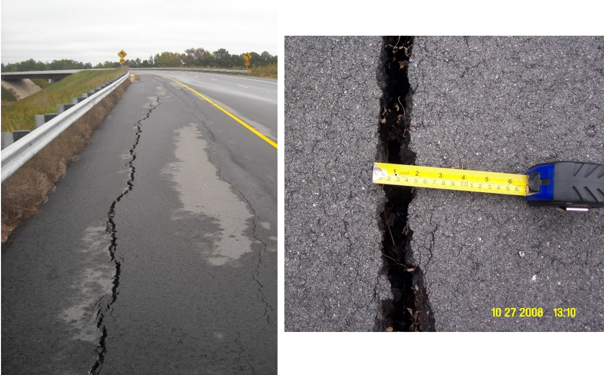
Figure 2.5. Longitudinal cracking caused by strength loss after wetting-drying cycles, NC I-540 @ Davis Drive (source: “Geotextile for Pavement Stabilization” presentation by NCDOT office)
