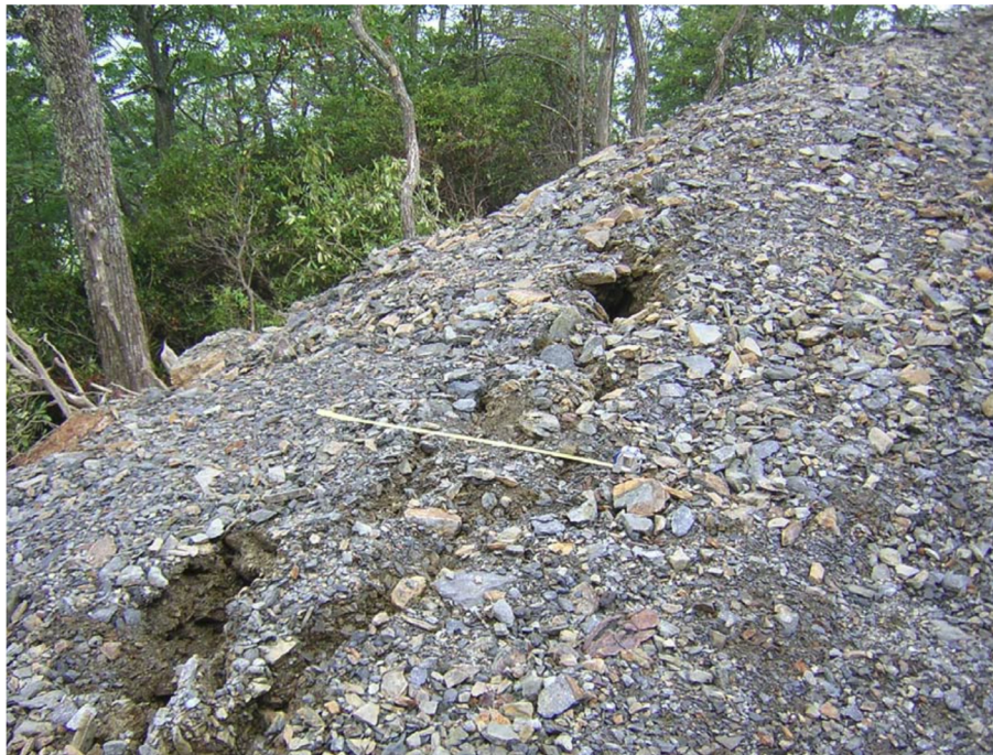
Figure 2.6. View of cracks in embankment, Haywood County, North Carolina (source: North Carolina Geological Survey 2006)
