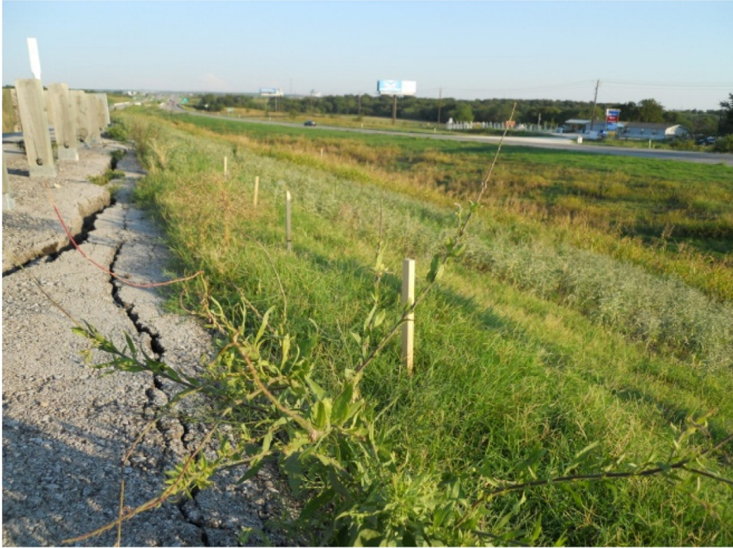
Figure 2.9. Surficial movement and cracked shoulder due to rainfall on U.S. Highway 287, Texas [photo credit: Khan et al. 2015]
