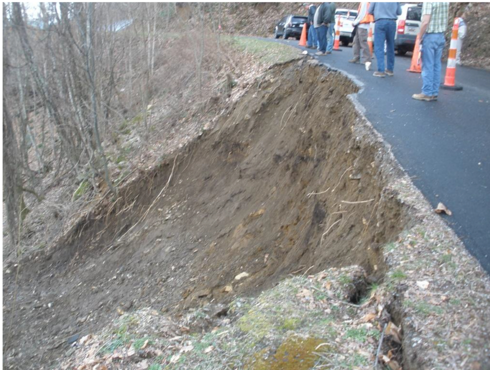
Figure 2.7. Embankment failure from the shoulder of roadway (Appalachian Landslide Consultants 2013)
