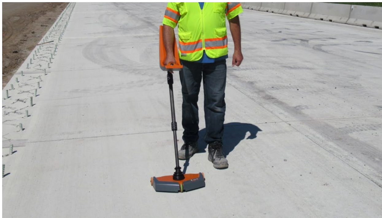
Figure 3. MIT Scan T3 operated on a new PCC pavement to determine thickness.
