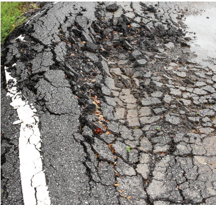
Figure 1: Example pavement cracking
