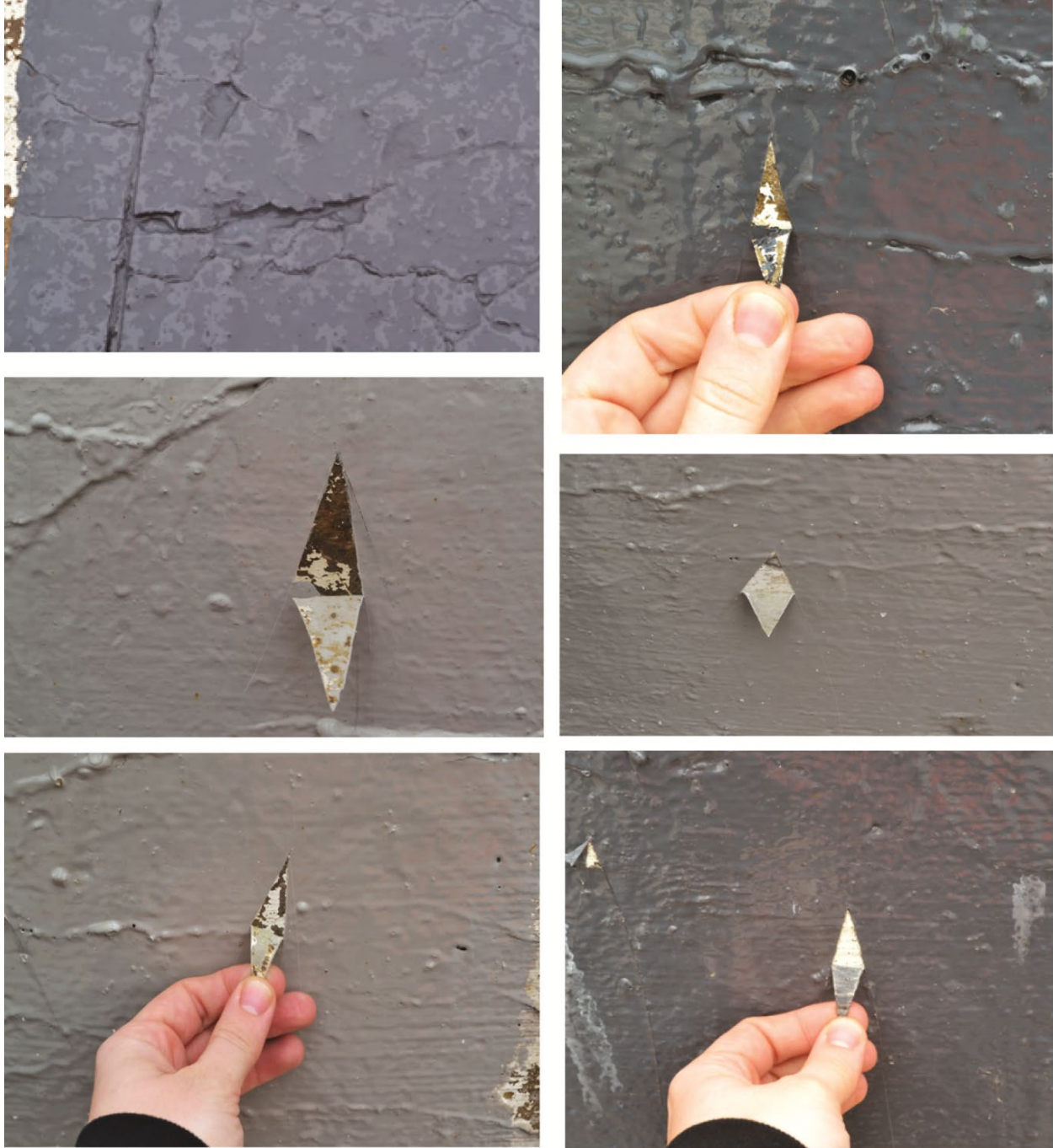
Figure 49: V-notch test on unprepped parapets with existing epoxy from Application No. 2 on Gantz Rd. Bridge
