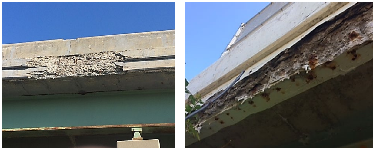
Figure 1: Example of the condition of a damaged parapet in District 6
