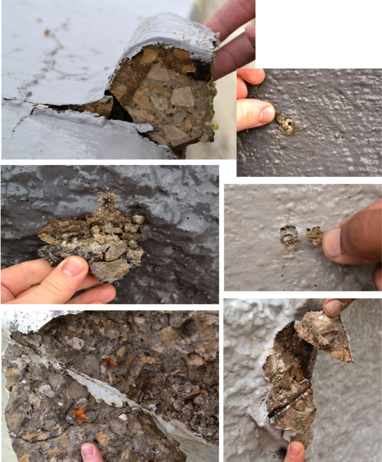
Figure 51: Impact test on parapets with existing epoxy from Application No. 1 on SR142 Bridge over I-70
