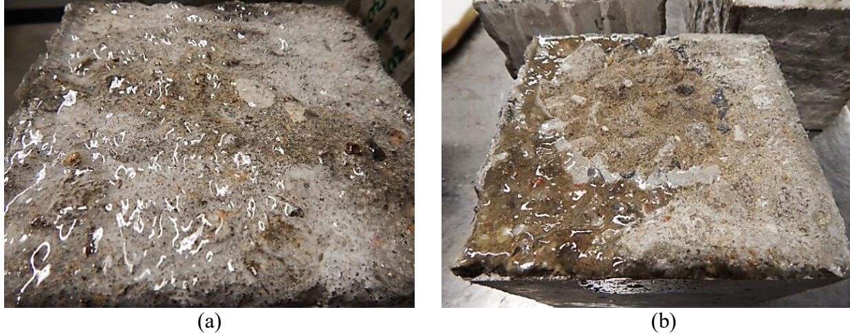
Figure 57: (a) Rust-Oleum RG-80X disbondment prior to testing flaking and (b) VersaFlex Clear Seal flaking from surface
