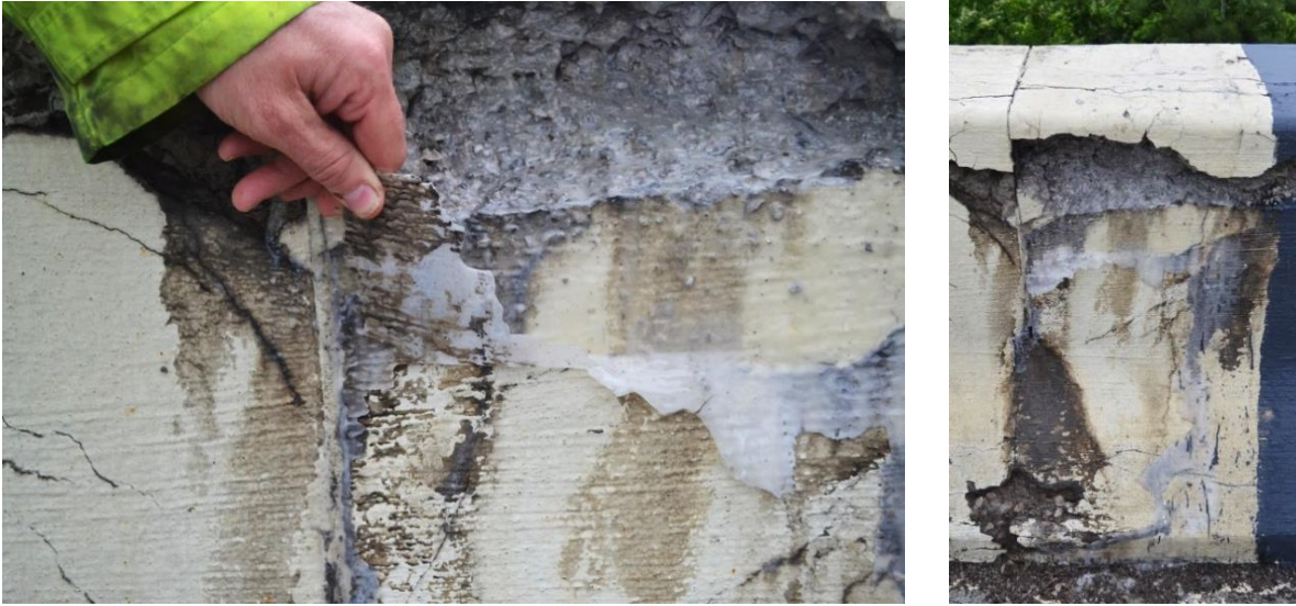
Figure 47: Failed product 5 of Application No. 2 on Gantz Rd. Bridge
