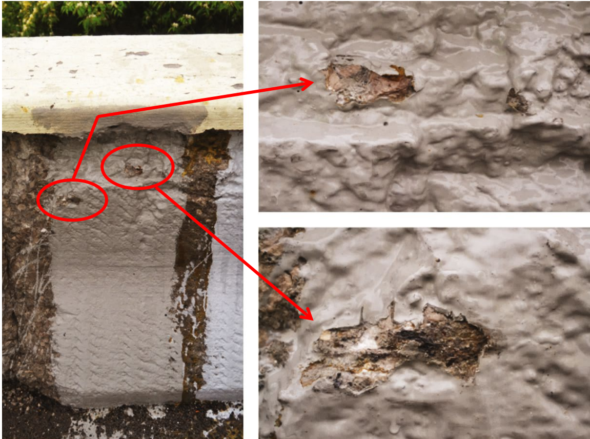
Figure 46: Product 1 substrate and polyaspartic coating failure
