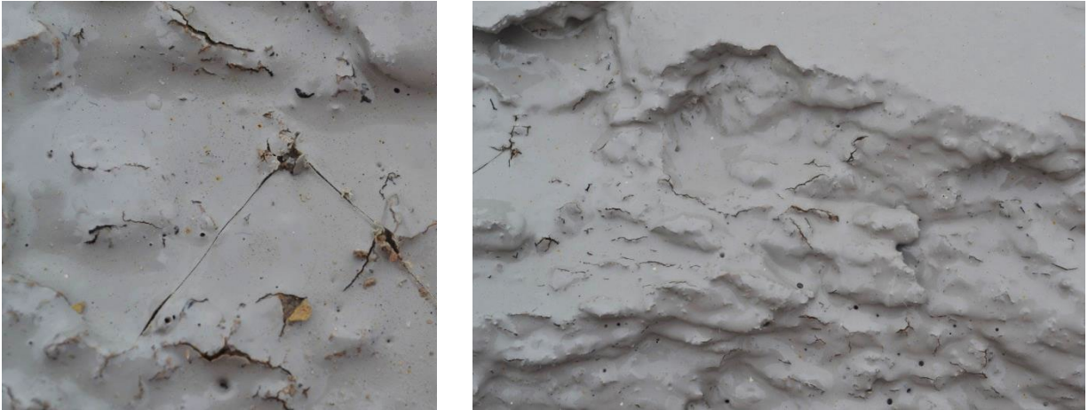
Figure 52: Small cracks observed in rough aggregate areas of the coated parapet walls
