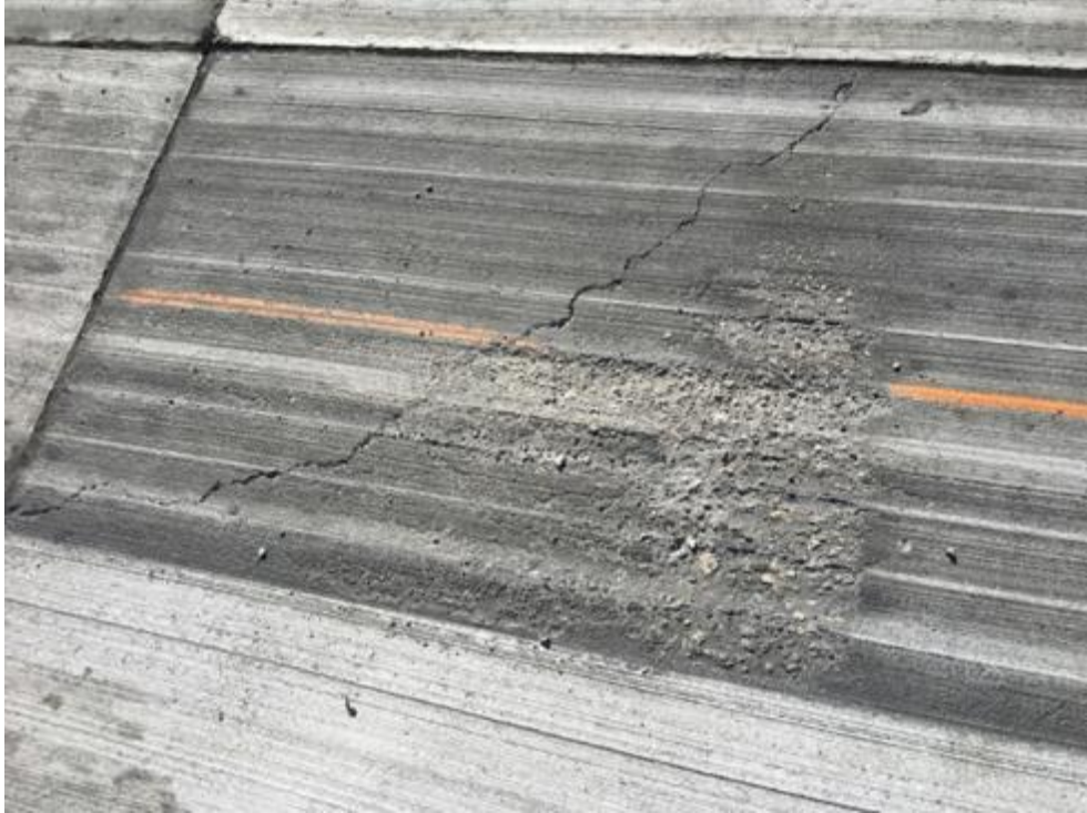
Fig 4.12 Surface of Slab2 ICC-2 after HVS loading.
