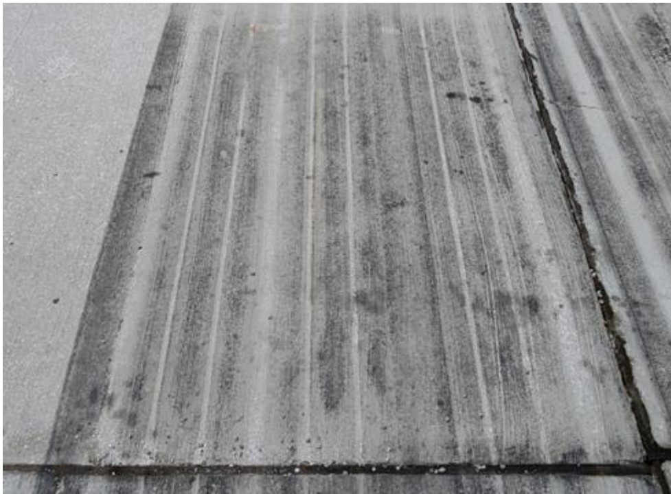
Fig 4.15 Surface of Slab4 SC after HVS loading.
