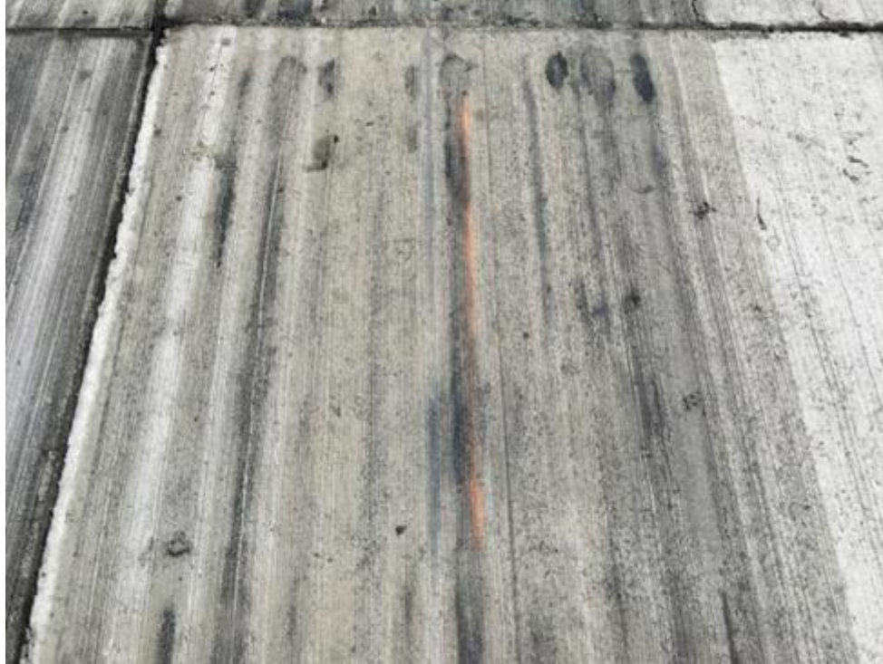
Fig 4.14 Surface of Slab1 ICC-1 after HVS loading.
