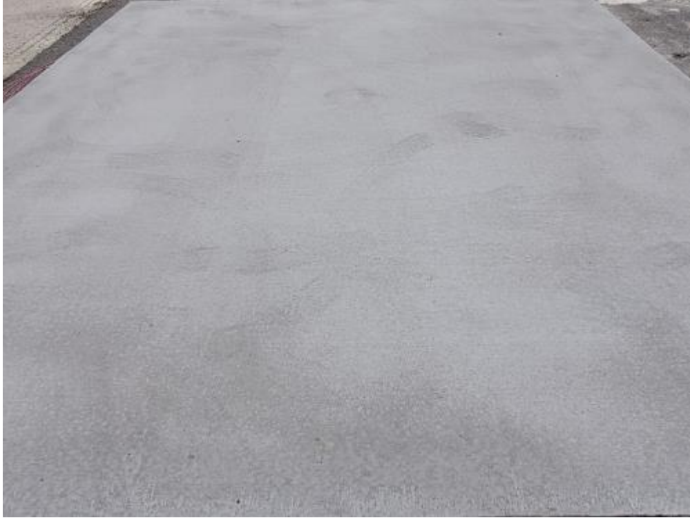
Fig 5.13 Picture of the surface of Slab2 ICC-1.
