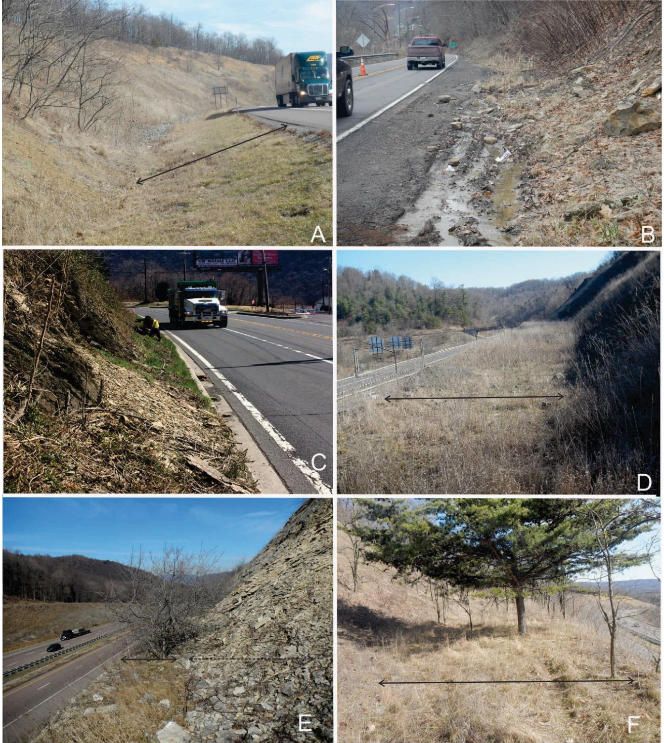
Figure 5. Benches and catchments styles and character. A, Catchment shoulder sloping away from roadway. B, Flat catchment shoulder. C, Shoulder inclined towards roadway. D, Elevated catchment bench clear of debris. E, Elevated bench nearly filled with debris. F, Elevated bench with woody vegetation.
