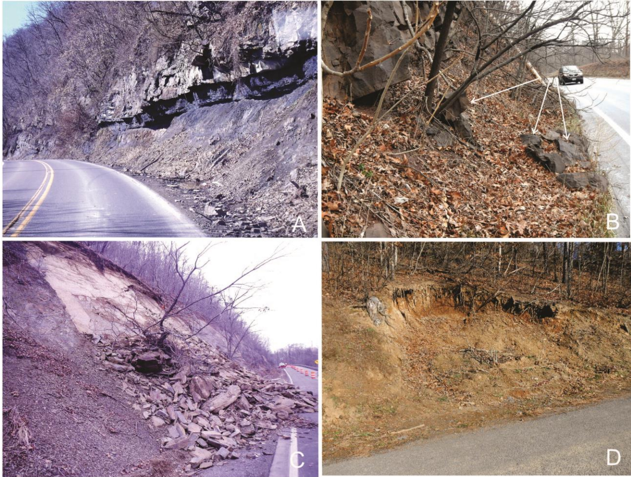
Figure 10. Type of slope failures and resulting hazards identified during this study. A, Rockfall. B, Rock roll. C, Rock slide. D, Slump (rotation) scar.
