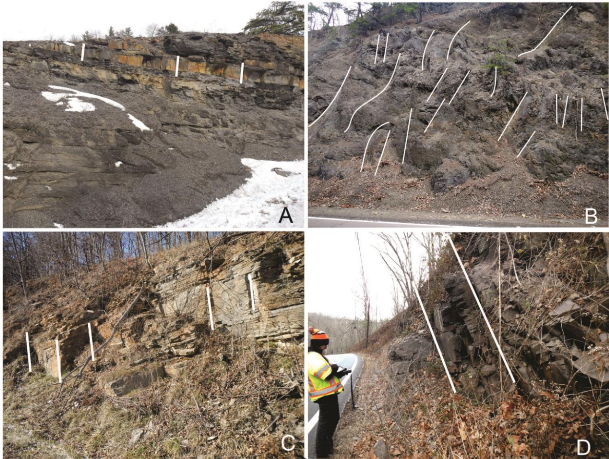
Figure 11. Failure plane character. A, Discontinuous and favorable orientation. B, Discontinuous and random orientation. C, Discontinuous and adverse orientation. D, Continuous and adverse orientation.
