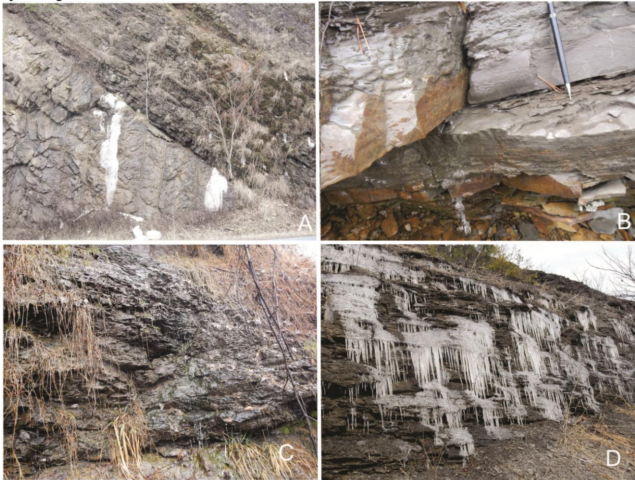
Figure 7. Degrees of variation in the amount and distribution of water on roadside slopes. A, Water seeps along stratification. B, Water seeping along joints and fractures. C, D, Water covering the surface of outcrops.
