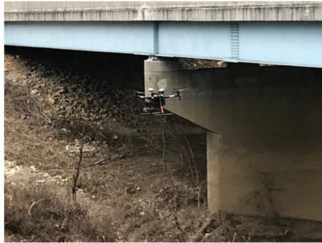
(b) UAS can document areas of bridge that are difficult to access (Fitzgerald, 2020).
