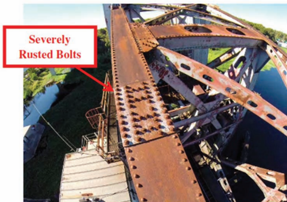
Figure 6.8 Rusted bolts on steel bridge detected by UAS (Otero et al., 2015).
