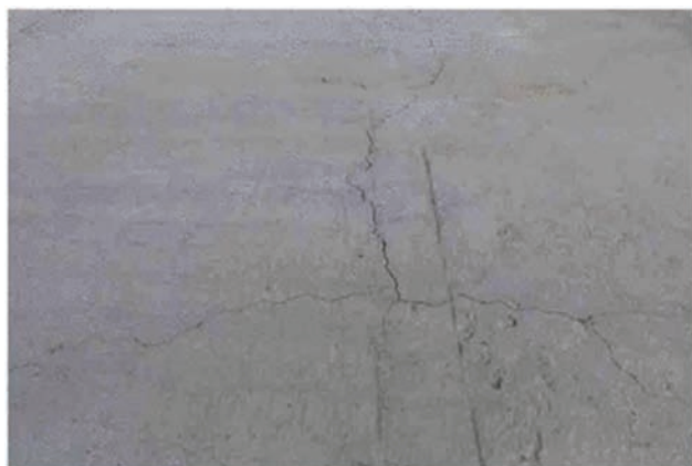
Figure 6.1 Cracks in pavement recorded by UAS (Dorafshan et al., 2017).
