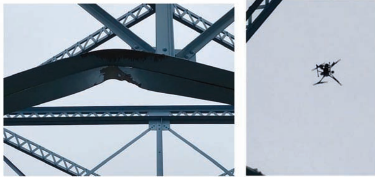
(a) UAS provides excellent vantage point to document bridge damage after bridge hit (Fitzgerald, 2020).
