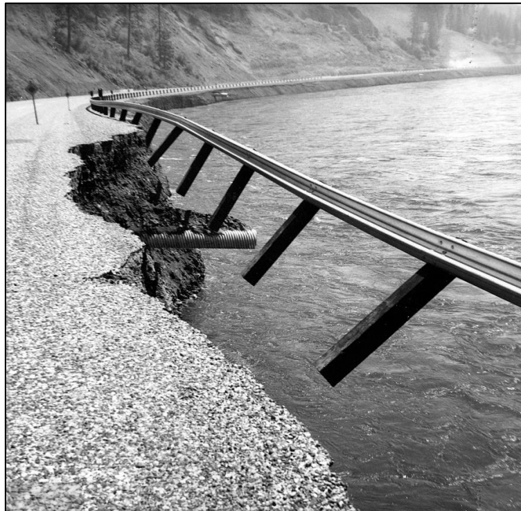
Figure 116. Flooding on US-12 near Kooskia in May 1964 washed out a portion of the highway and guardrail. 573
