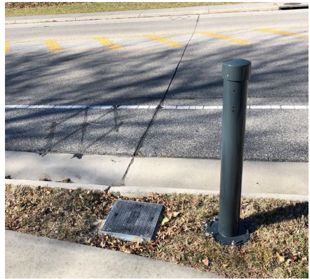
Figure 3: Completed installation using cut-in inductive loops at Tom's Creek Road in Blacksburg, Virginia. (Image courtesy of Virginia Department of Transportation)
