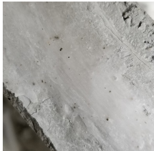
(b) Example of a crack from the top view
