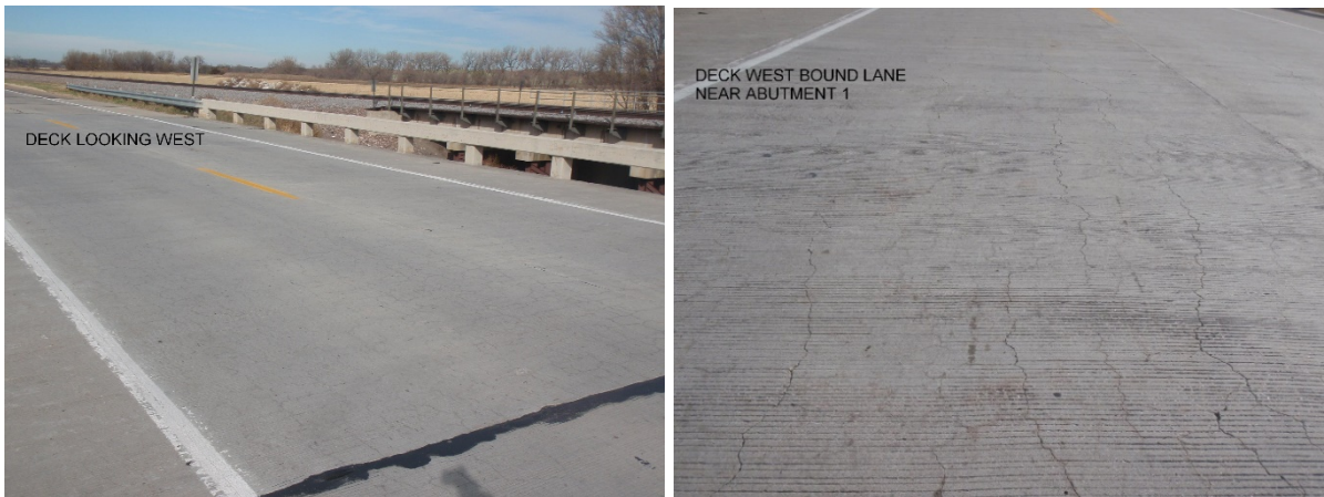
Figure 1. Examples of bridge deck cracking (photos from NDOT Bridge Inspection Database)
