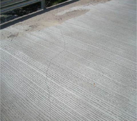
(a) Crack on a plain bridge deck
