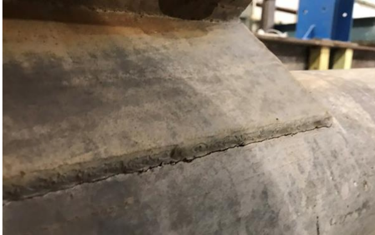
Figure 40. Fatigue crack in welded connection between reaction box and straight pole
