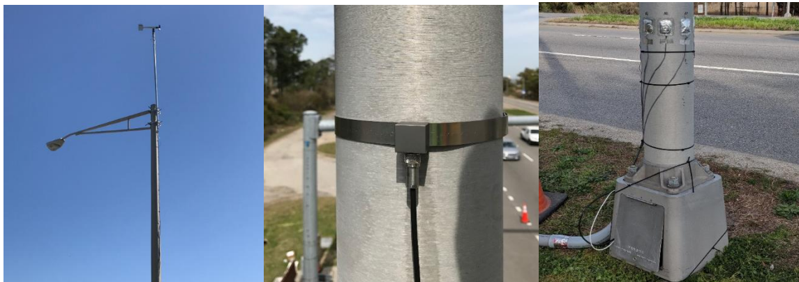
Figure 7. Wind monitor (left), accelerometer (center), and strain gages (right)
