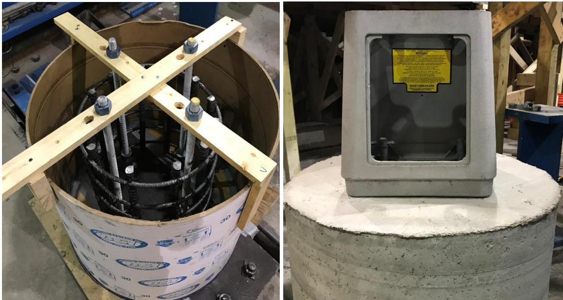
Figure 22. Formwork for the concrete foundation (left) and T-base with the casted foundation (right)
