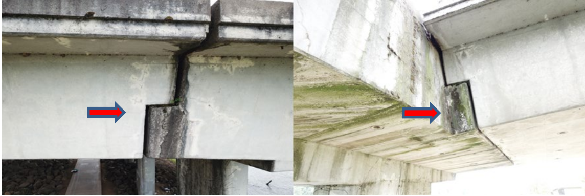
Figure 5.3 A failed joint seal leaking water
