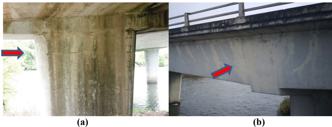
Figure 5.1 (a) Hairline shrinkage cracks on a column; (b) Hairline flexure cracks with efflorescence on the sides of boxes
