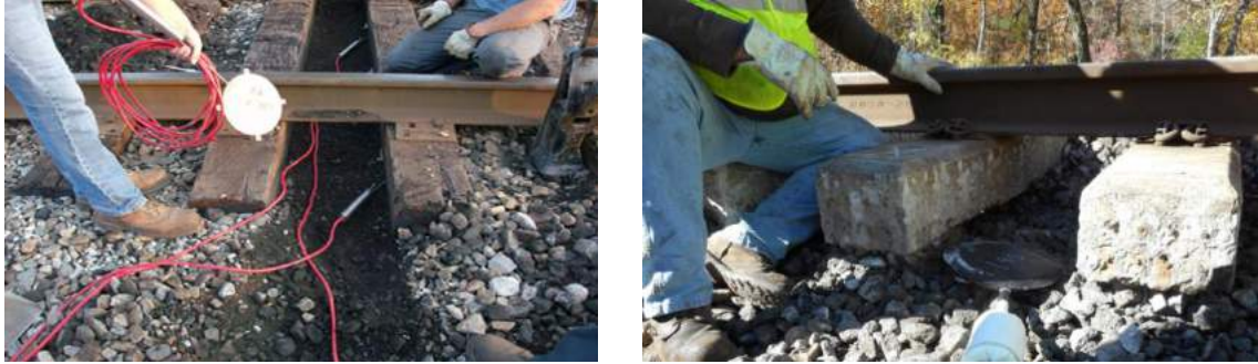
Figure 2. Two track sites used for initial attempts to accurately measure tie/ballast interfacial pressures, TTI Railroad yard lead (left) and NS mainline (right).
