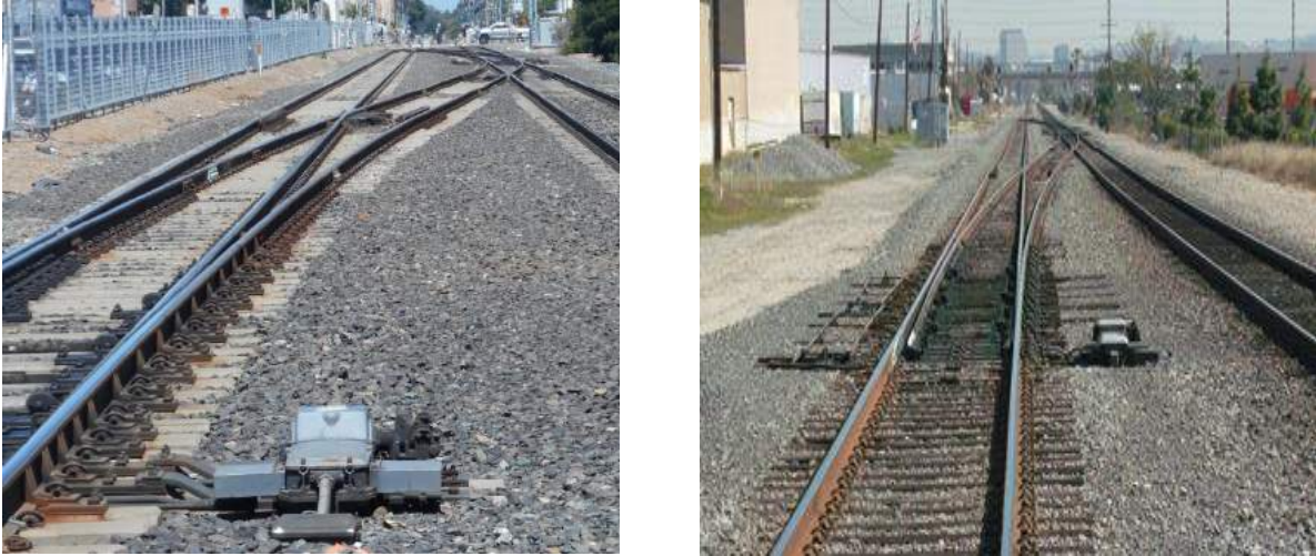
Figure 5.1. Views of a Universal Crossovers on Caltrain at CP Palm (left) and on Metrolink's Antelope Valley Line (right). These Crossovers have been Maintenance Free for Many Years.
