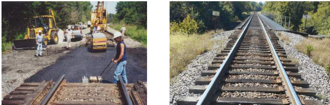
Figure 6.2. Renewal process for Approach to a Short Open-Deck Bridge on CSX Line near Ft. Estill, KY (left) and condition after 15 years of Traffic (right).
