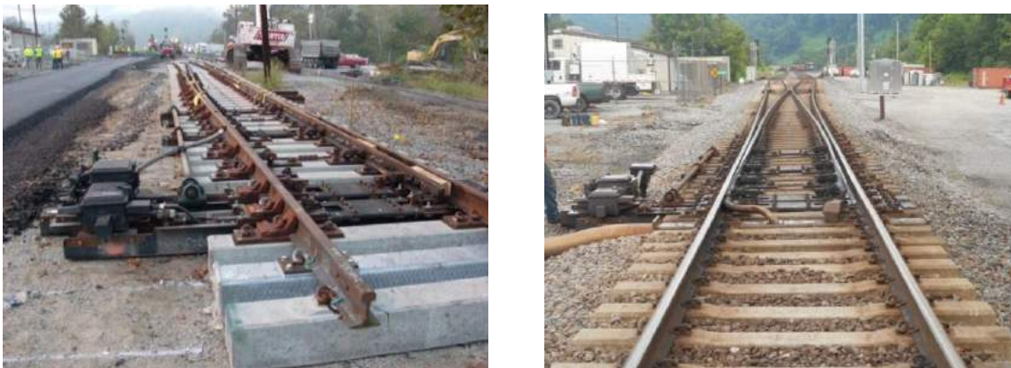
Figure 5.3. A No. 20 Equilateral Turnout at Greyeagle, WV before positioning on the Asphalt Pad on left which had been placed earlier that morning and after four years of traffic on right.
