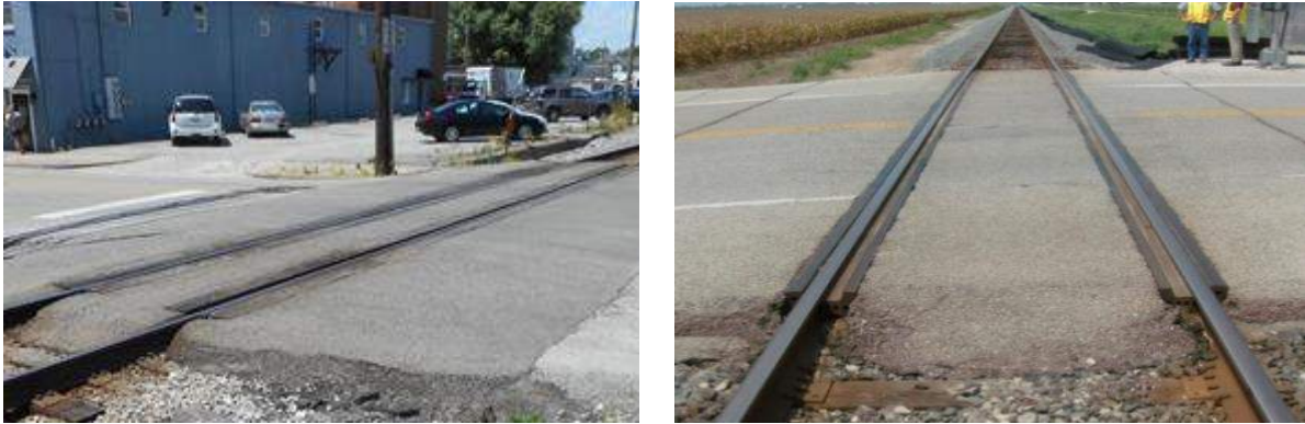
Figure 3.9. Pike Street Crossing (left) in Cynthiana, renewed with Asphalt Underlayment in 1984, Surface replaced twice during the 32 intervening years. US 60 Crossing (right) at Stanley, ten years after renewal with Asphalt Underlayment, Still in perfect condition in 2012.
