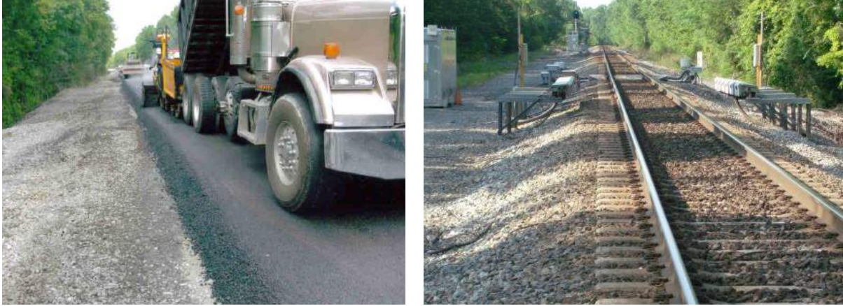
Figure 8.1. Asphalt Paving in preparation for installing the Salient Process WILD on NS Line at Flatrock, KY in 2009.
