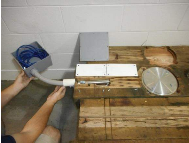
Figure 6.2a. A typical routed tie with a recess and a pressure cell.
