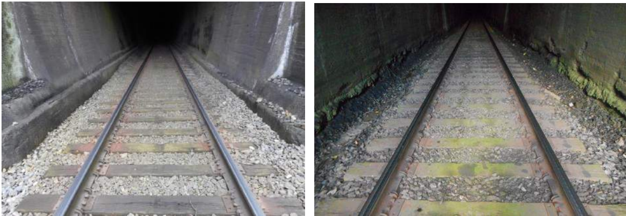
Figure 7.1. Vasper Tunnel (left), 1500 ft (457 m) has been Dry all the way through only requiring maintenance surfacing for crosslevel twice during Five-Year Spans. Similar success for the Cove Lake Tunnel (right), 1750 ft (533 m) except for a couple of waterfalls requiring maintenance to periodically clean the ditches. Both are on the KD Subdivision.
