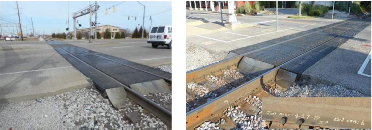
Figure 3.6a. Charlestown-New Albany Road Crossing in Jeffersonville (left) installed in 2003; State Route 256 Crossing in Austin (right) installed in 2007, Recent Rail Upgrade is shown on Left Bottom, (inset bottom right shows Sept. 2015 Weld), the 9-Year Old Existing Crossing was Unaffected.
