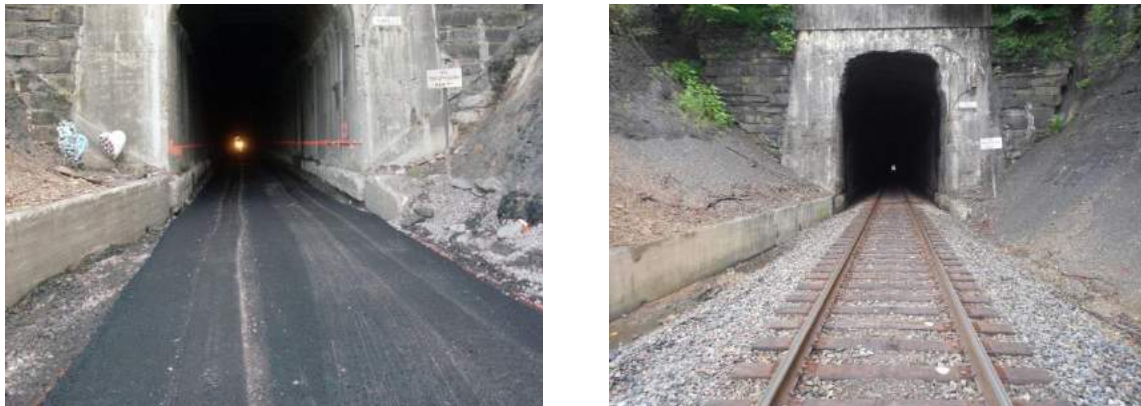
Figure 7.2. Big Sandy Tunnel No. 3 near Greyeagle, WV with the paved trackbed during the Tunnel Clearance Project in 2010 and the finished approach to the Tunnel in 2016. Maintenance costs have been minimal since 2010.
