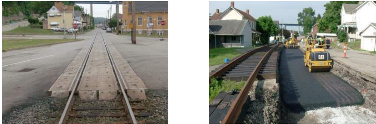
Figure 9.2. Main Street Paved Trackage in West Brownsville, PA. The earliest placed section after five years of traffic (left) and paving one of the sections within the excavated trench (right).
