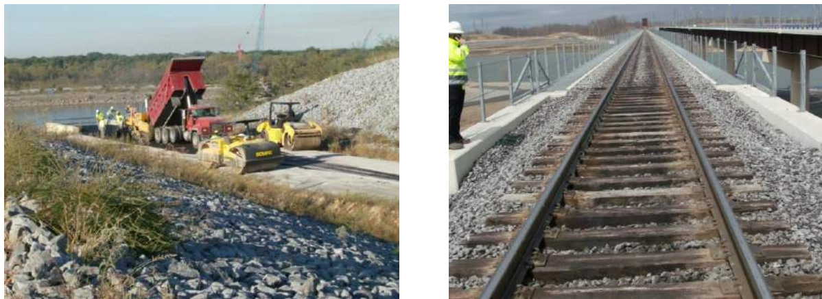
Figure 6.3a. Paving the North End Approach prior to erecting the Bridge (left) and a recent view of the West End of the Kentucky Dam Bridge (right).
