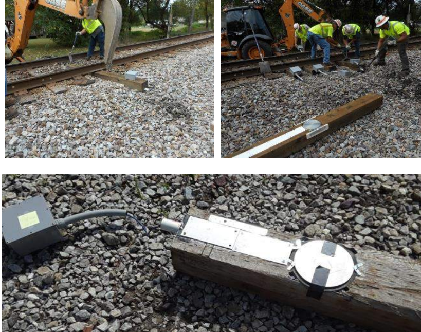
Figure 5a. NS crews inserting instrumented ties in the trackbed at Mascot. The bottom view is an instrumented tie prior to installing in the track. The recessed cell will be on the bottom of the tie, level with the surface of the ballast.
