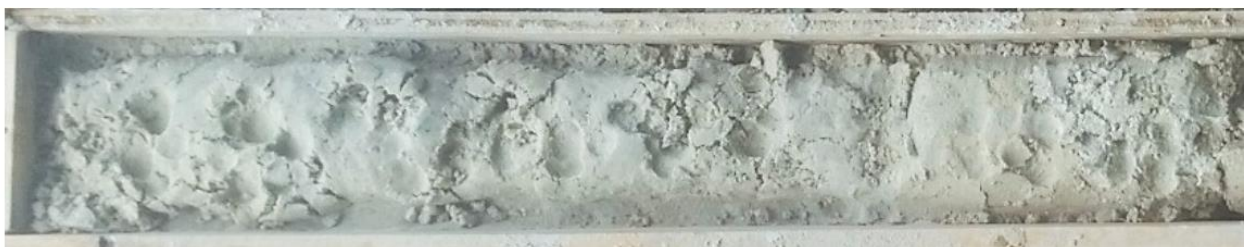
Figure 2-5. Weak, poorly cemented silt, sand, and limestone mixture in a core run
