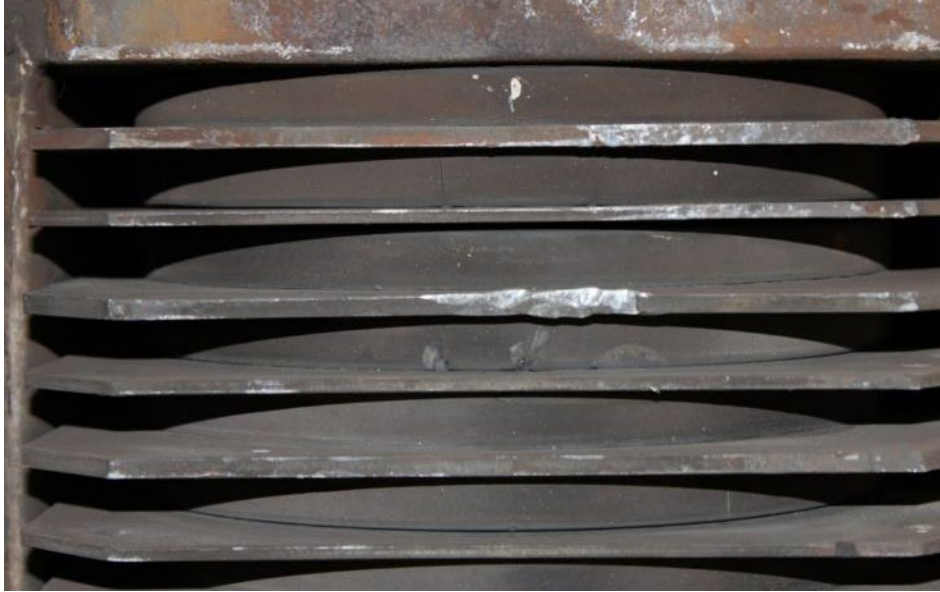
Figure 33. Chipped Draft Plate
