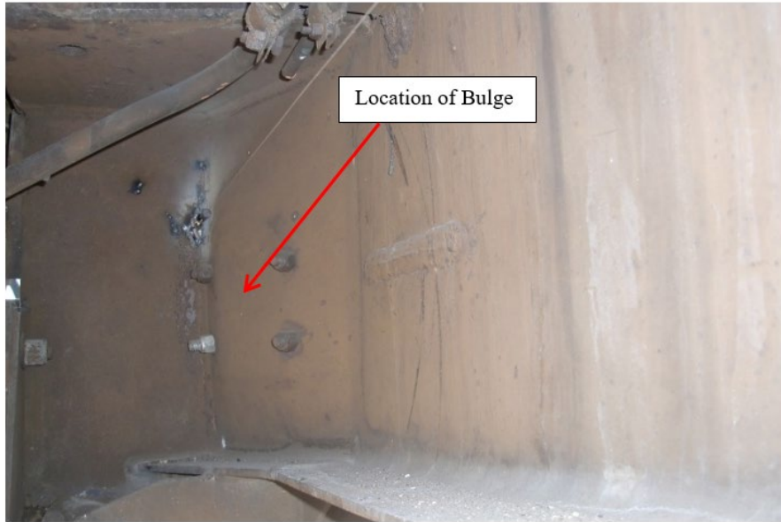
Figure 39. Draft Pocket Side Wall Bulge
