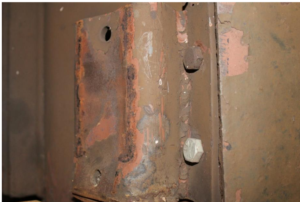
Figure 38. Damaged Buff Stop
