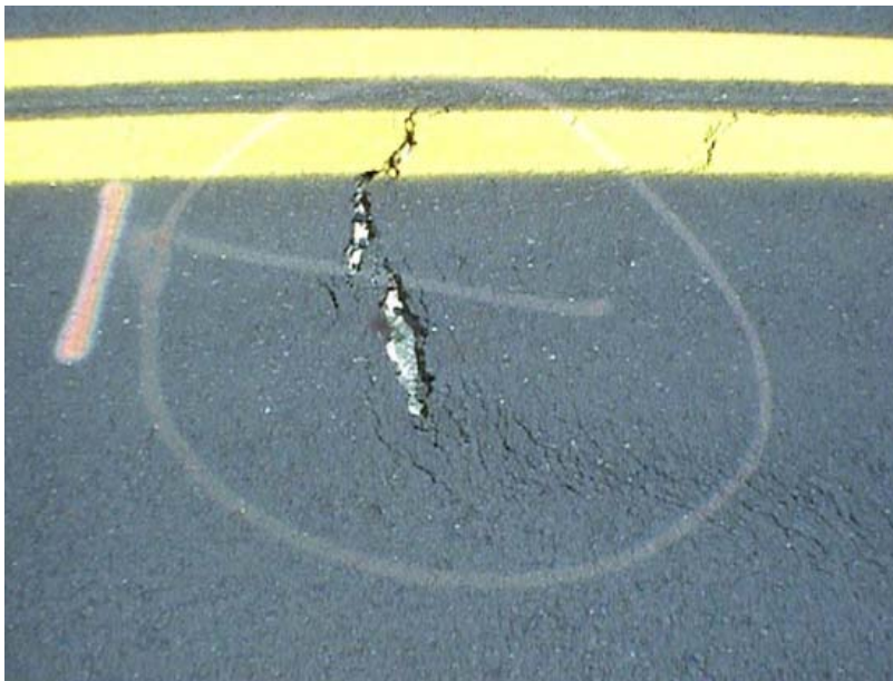
Figure 19. Cracking and Delamination on CR 315 (Sholar et al., 2002)
