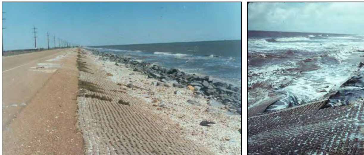
Figure 7.21. Example of failed block revetment (Louisiana SH 82, circa 1980, USACE archives photos)
