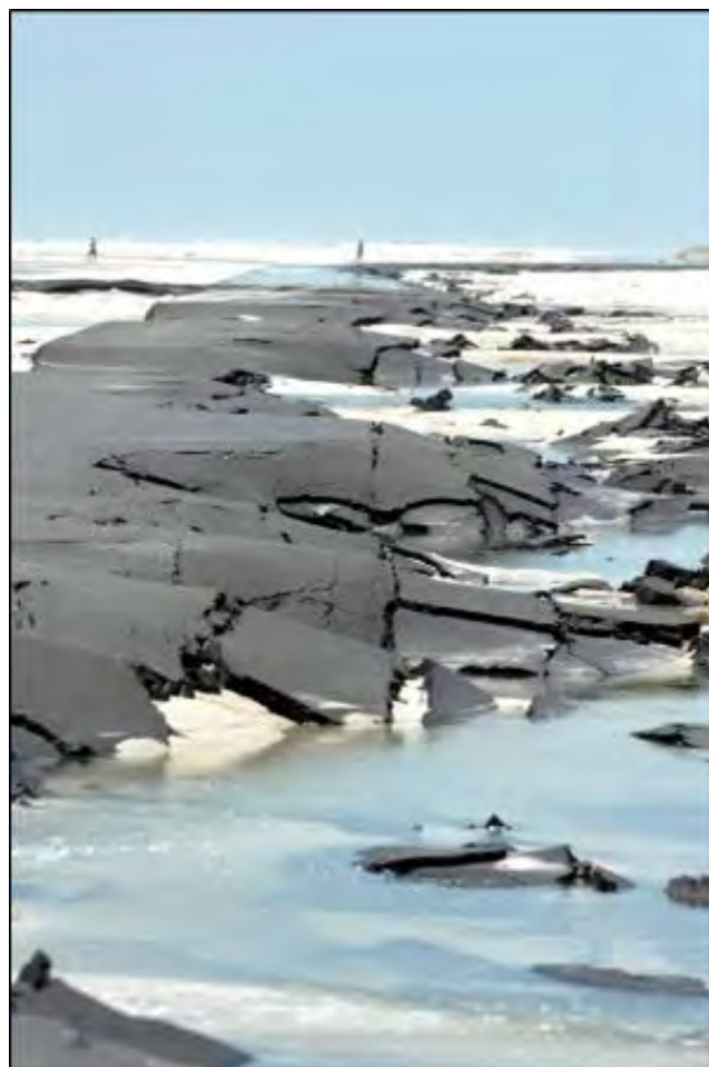
Figure 10.5. Pavement destroyed by the weir-flow mechanism (Fort Pickens Road, Gulf Islands National Seashore, near Pensacola, Florida)
