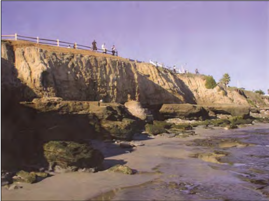
Figure 7.13. Concrete seawall designed to look like the natural rock formation built on an eroding sea cliff to protect a local road (East Cliff Drive, Santa Cruz, California, 2001)
