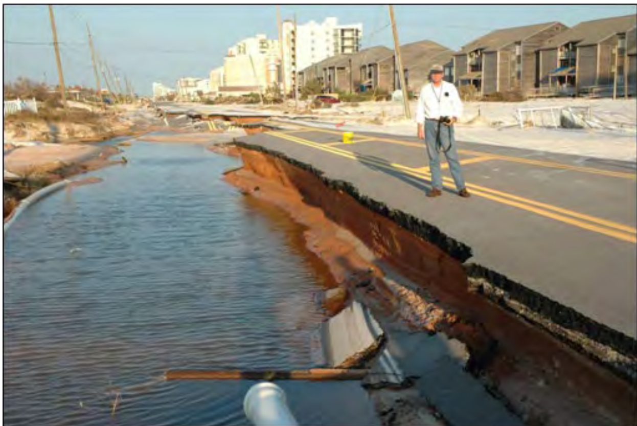
Figure 10.1. Example of pavement damage due to storm surge (Florida SH 292 on Perdido Key after Hurricane Ivan, September 2004).
