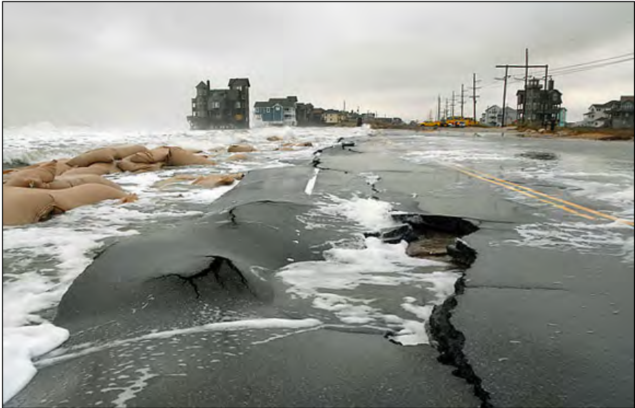
Figure 15.4. Pavement damage due to waves and surge in an extreme event (North Carolina SH 12, 2009; permission to use photograph provided by Dave Henderson)
