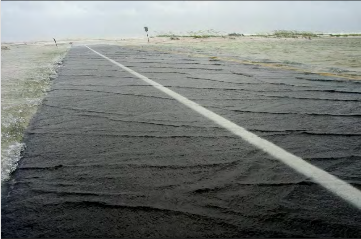
Figure 10.6. Weir-flow damage beginning (Fort Pickens Road, Gulf Islands National Seashore, Florida, July 2005; FHWA photograph)
