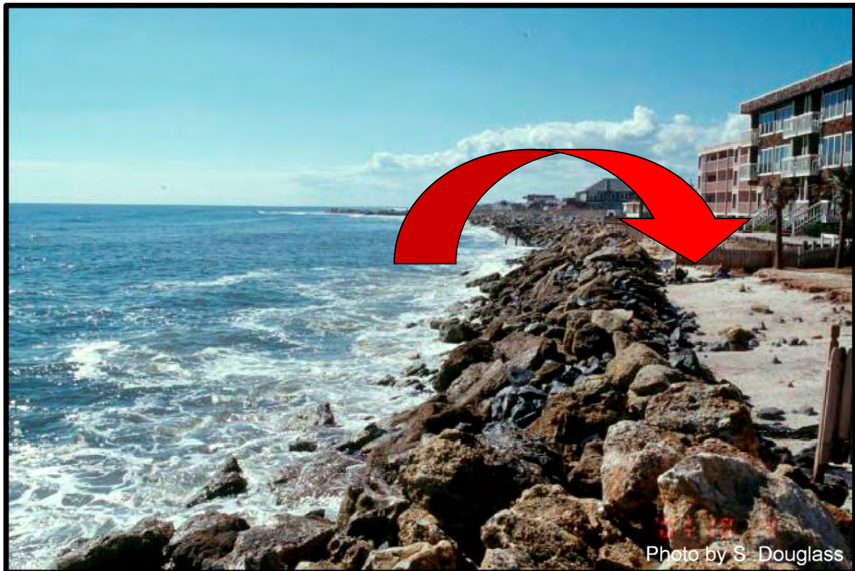
Figure 7.18. An example of splash damage behind seawall (circa 2004)
