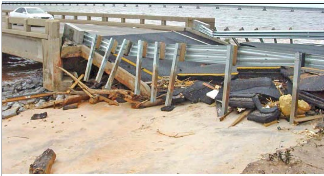
Figure 12.19. Damage to bridge approach behind abutment due to wave action in a hurricane
