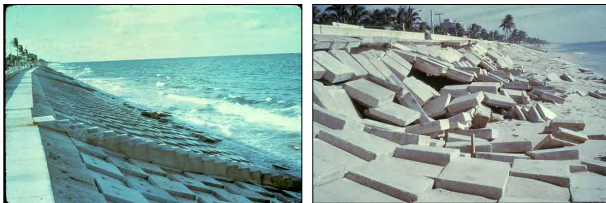
Figure 7.20. Example of rigid concrete-block revetment failure (Florida SH A1A, Delray Beach, circa 1972; University of Florida and USACE archive photos)
