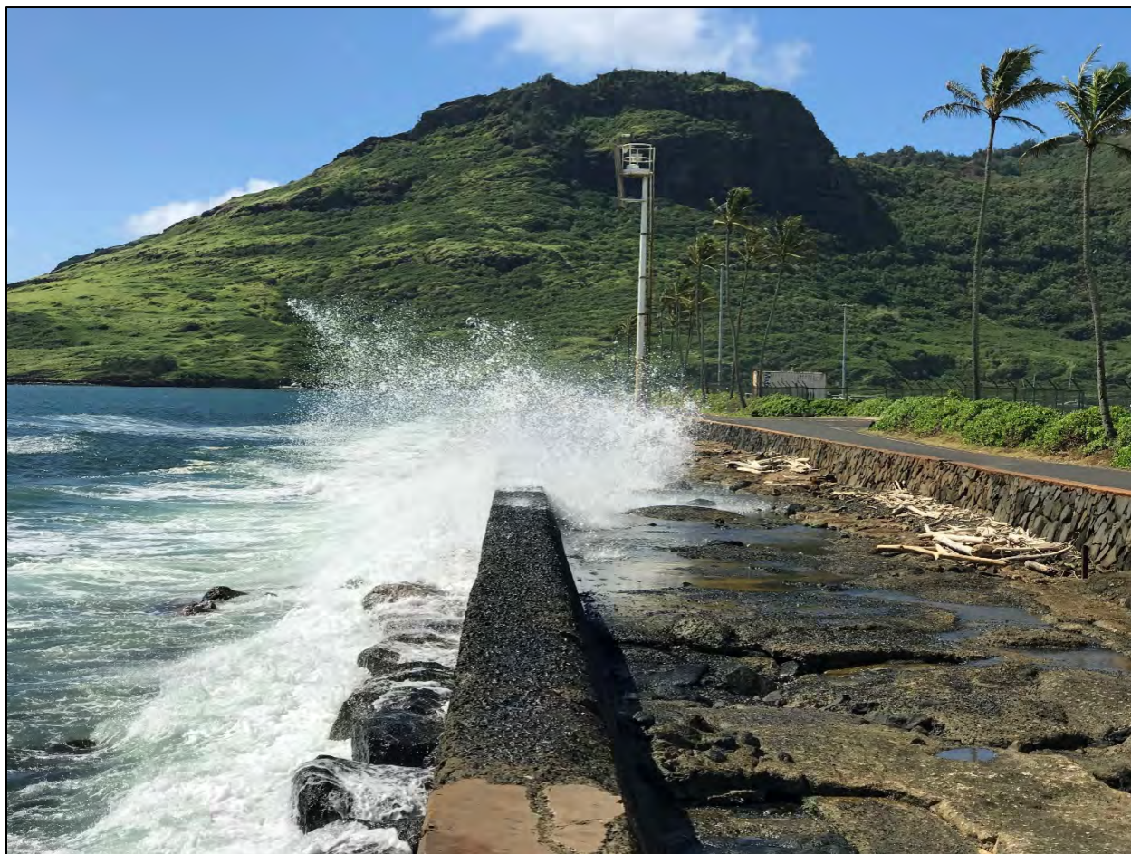
Figure 7.23. Wave overtopping a seawall (Lihue, Hawaii, 2018)
