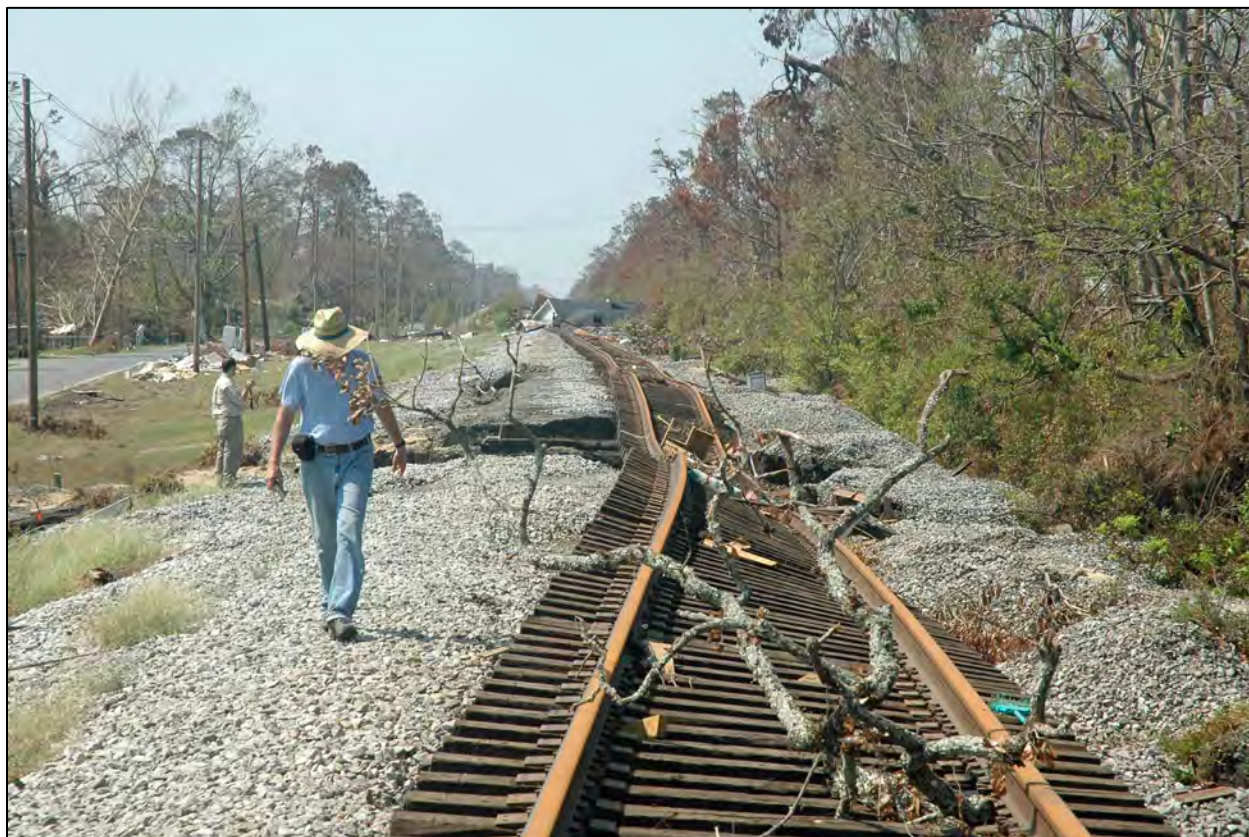
Figure 15.3. Railway embankment damage caused primarily by the coastal weir-flow damage mechanism during (Mississippi, 2005)
