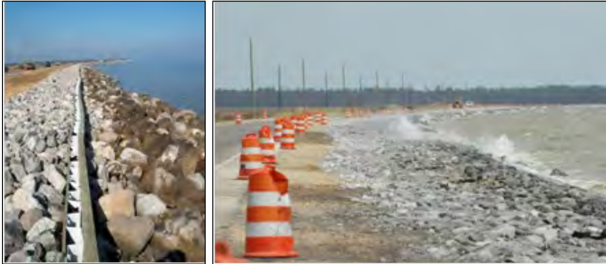
Figure 7.16. A revetment with rocks too small to withstand the wave attack at this location
