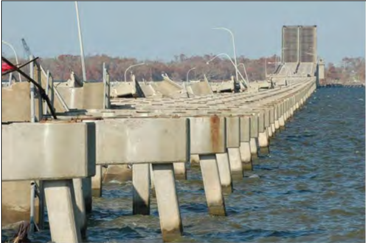
Figure 3.4. US Highway 90 bridge across Biloxi Bay, Mississippi, after Hurricane Katrina. (photograph looking northeast from Biloxi September 21, 2005)
