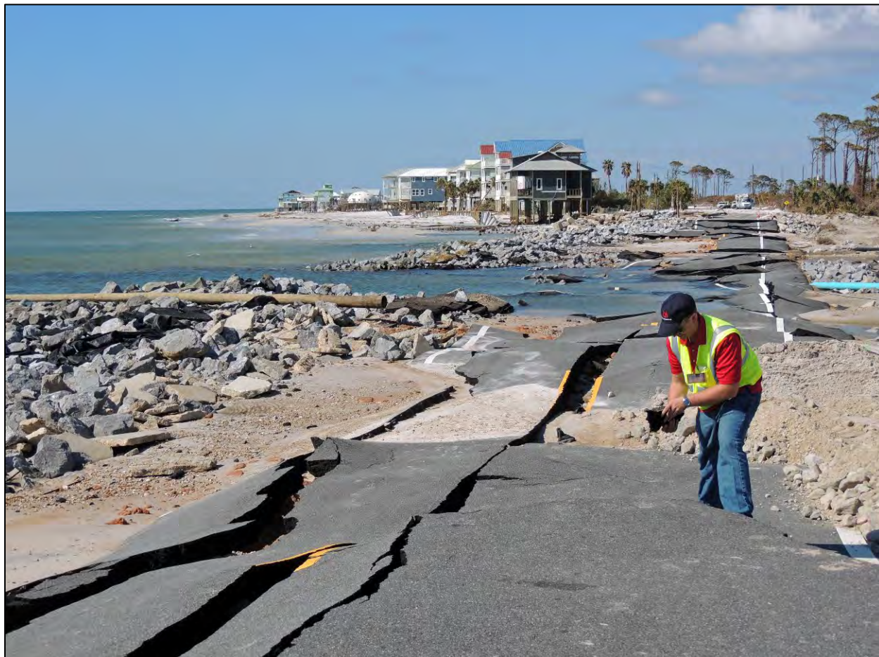
Figure 3.3. Damage caused by surge and waves in Hurricane Michael (October 14, 2018; permission to use photograph provided by John Cleary)
