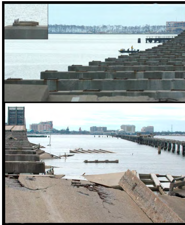
Figure 11.10. Details of damage to US 90 bridge over Biloxi Bay caused by Hurricane Katrina
