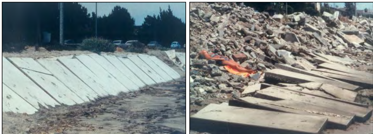
Figure 7.17. Example of a failed attempt at embankment protection (USACE archives photographs)
