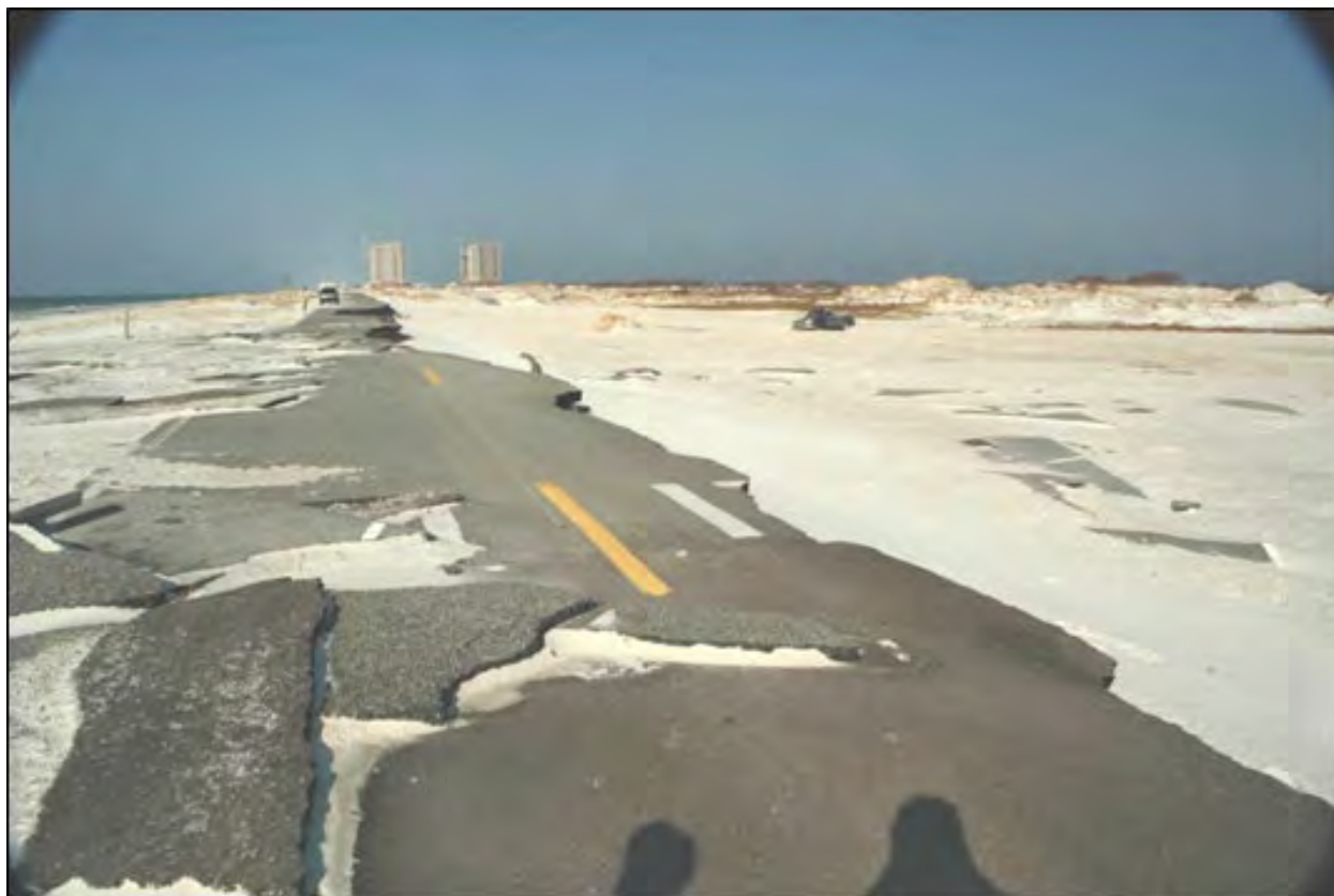
Figure 10.2. Example of pavement damaged by hurricane (photograph looking west on Florida SH 399, Gulf Islands National Seashore, 2005)
